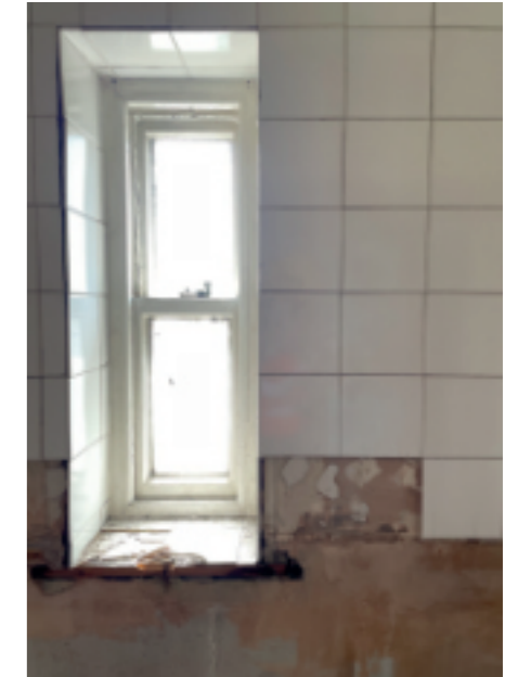
Dilapidated internal finishes
