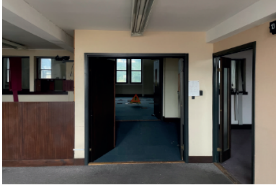
Ramped entrance to Computer Hall
