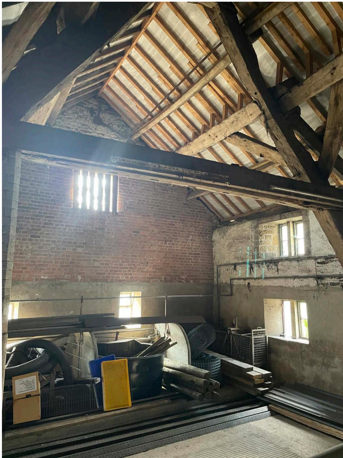
Photo Ref: E08 View of Nether Mill Barn (Internal Detailing Cruck Frame)
