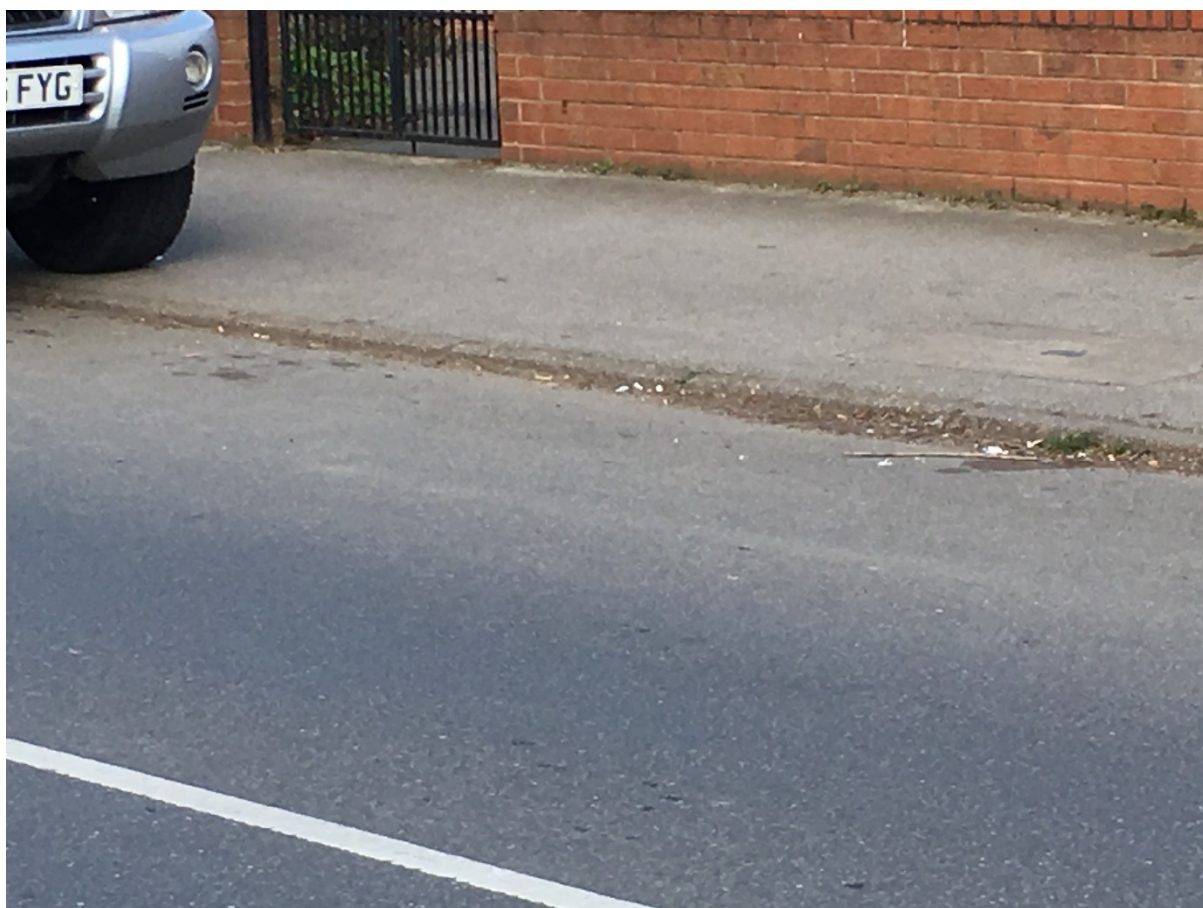
Figure 7 General road and kerb condition
