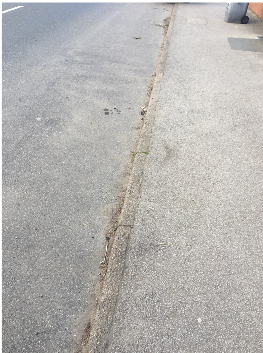
Figure 8 General condition showing areas of patching in footway
