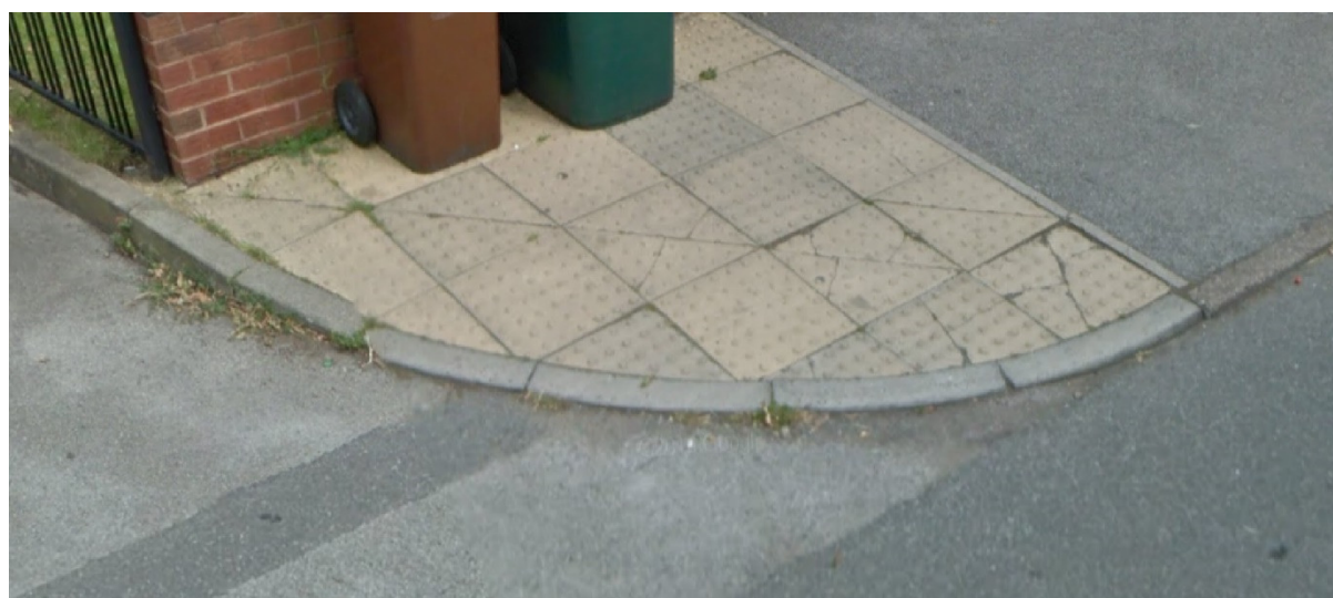
Figure 9 Tactile pavements showing signs of degradation
