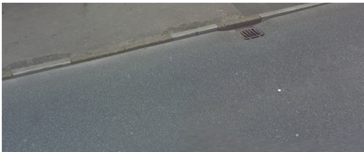
Figure 6 Sunken Road Gully
