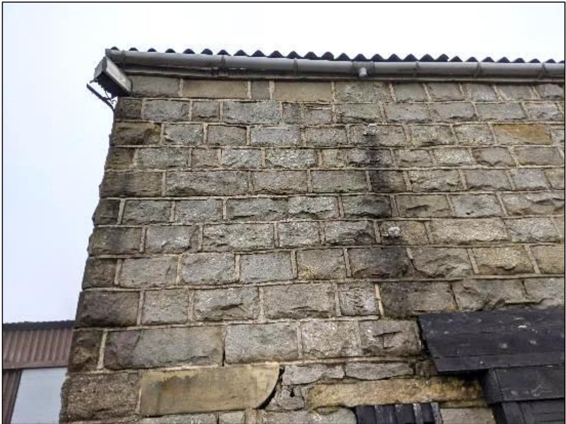
Plate 6. Section of south elevation of B3 with gaps between masonry and behind timber fascia both visible
