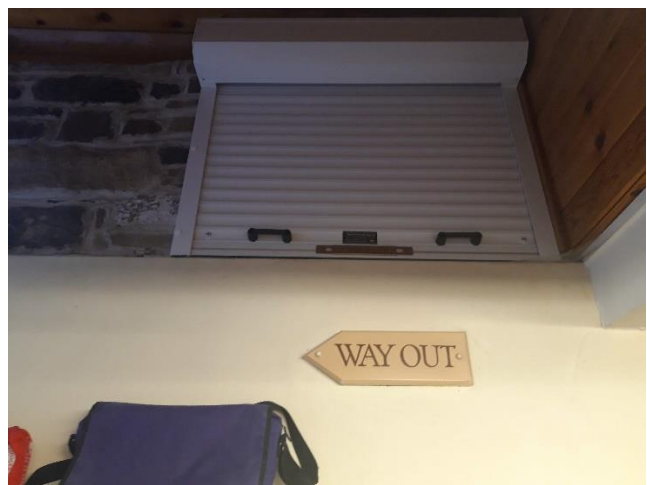
Mill Cottage: Security shutter on 0/001
