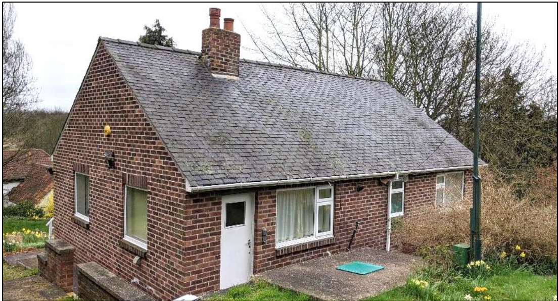
Plate 3. Missing ridge mortar adjacent to southeast gable
