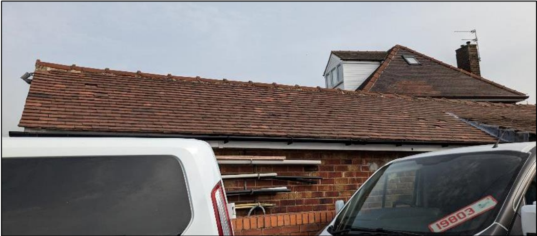
Plate 3. Missing plain tile on garage roof
