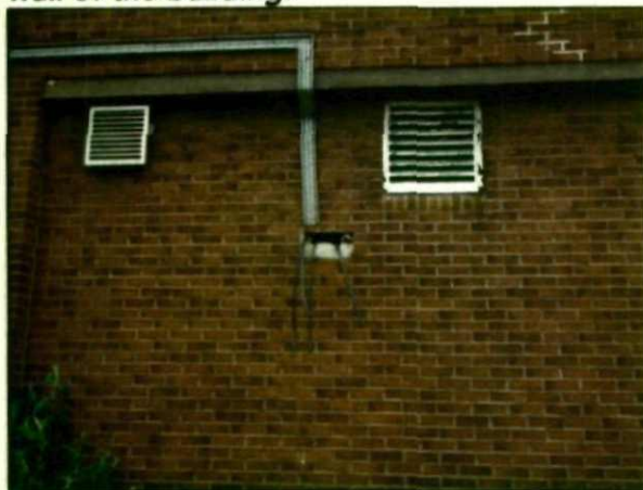
Figure 11: One of several holes in the east wall of the building.
