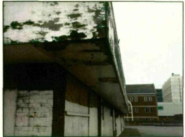
Figure 10: A gap in the boxed eave of the escalator well.
