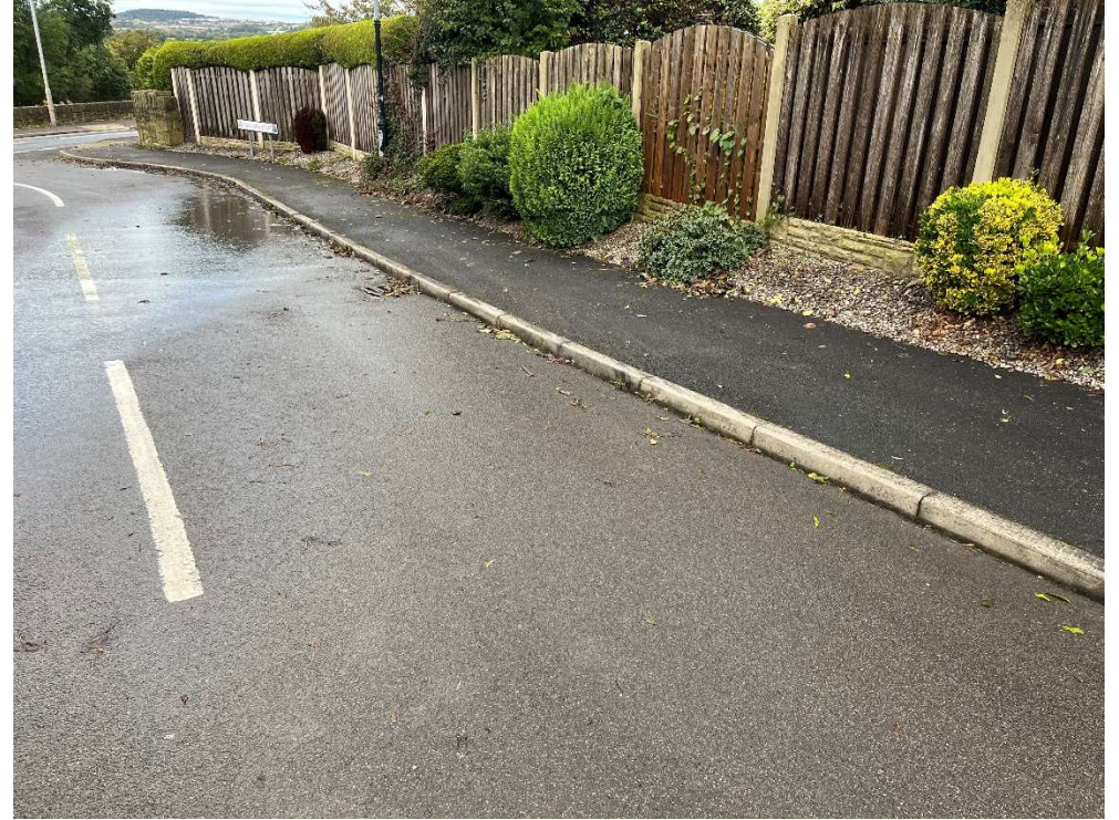
Balk Farm Court left side kerb opposite site entrance
