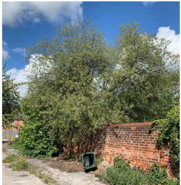
Figure 4: G4 and T5 growing either side of a brick wall to the north of the site.
