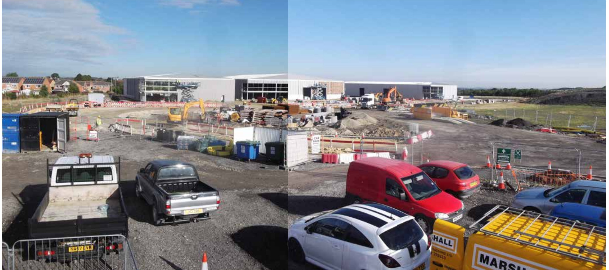
Fig.5 View from the site entrance looking towards the construction of Unit 2, 3 and 4
