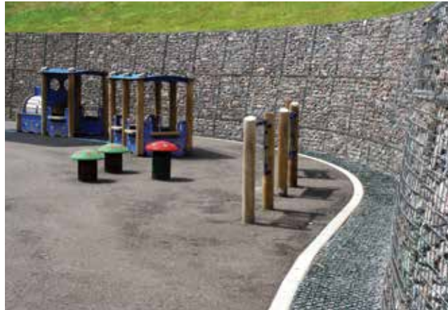
Figure 16.3 Filter drain with exceedance event managed within play area, Exwick, Devon (courtesy Robert Bray Associates)
