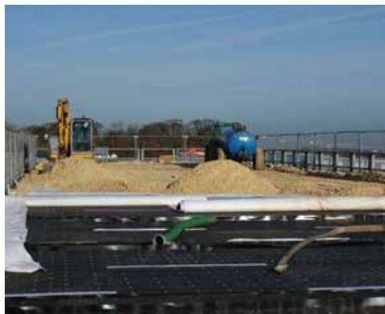
Figure 20.11 Construction of attenuation and irrigation system used below equestrian surfacing (courtesy Andrew Bowen)
