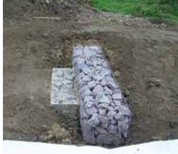
Figure 8.8b Check dam in a swale during construction, Lincoln (courtesy Lincolnshire County Council)
