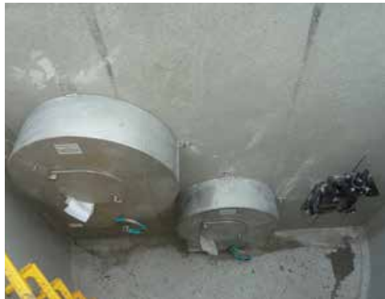
Figure 28.26 Two passive devices for multiple flow control (courtesy Hydro International)
