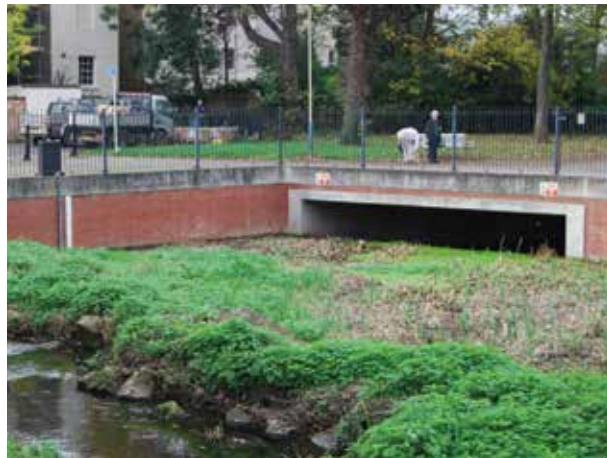
Figure 28.11 Example of landscaped flow splitter structure, River Chelt (courtesy Illman Young)
