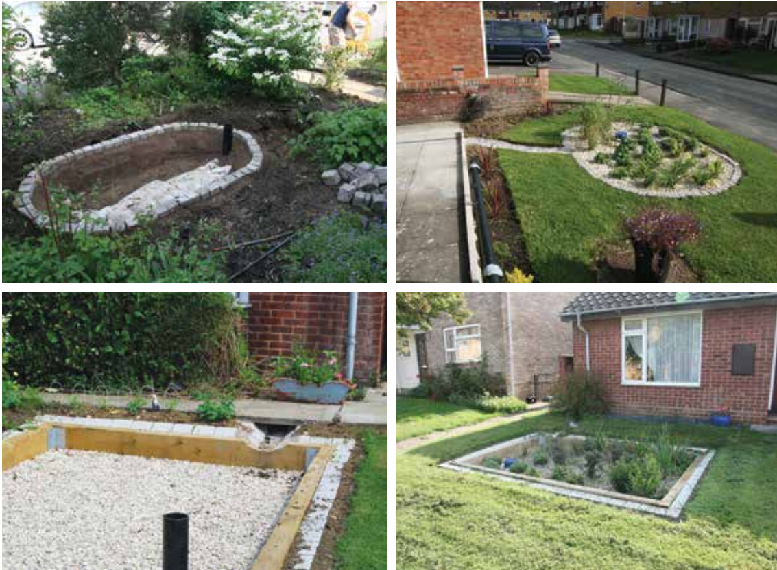
Figure 18.3 Examples of rain gardens under construction and planted, Cheltenham (courtesy EPG Limited and Illman Young)
