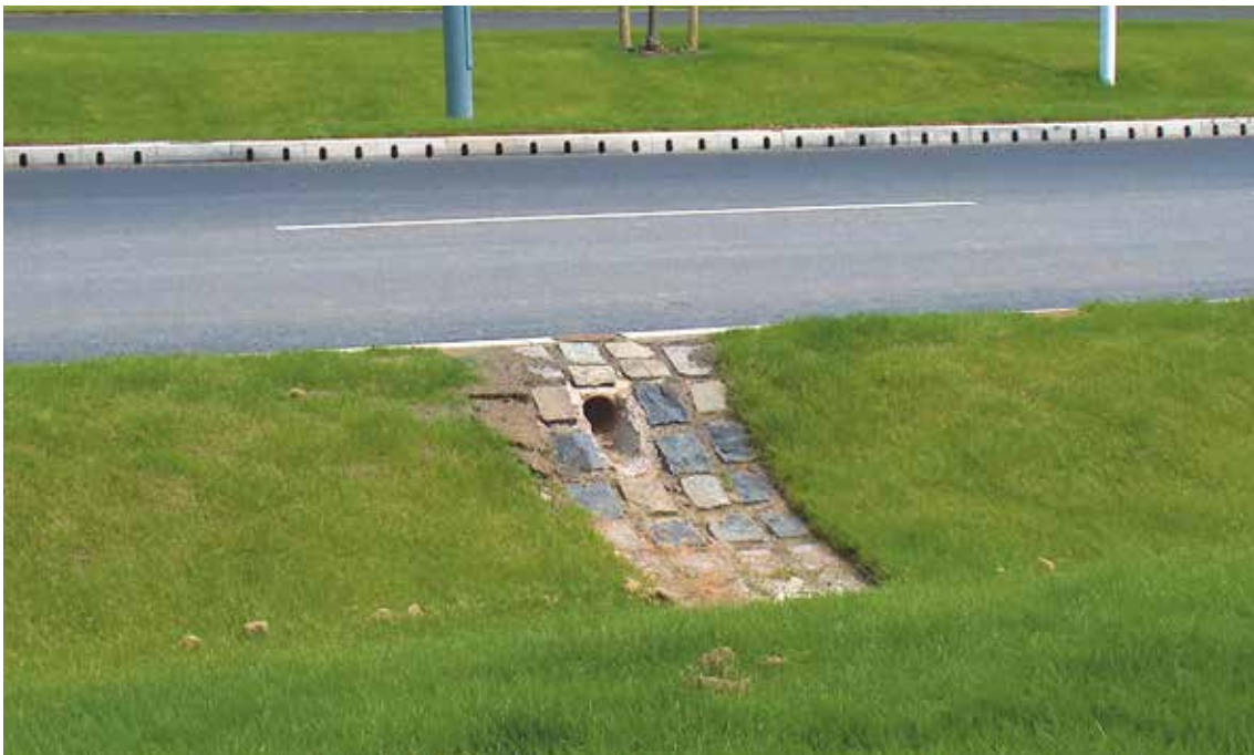
Figure 28.7 Kerb collection system being used to drain a carriageway in conjunction with a swale (courtesy ACO Limited)
