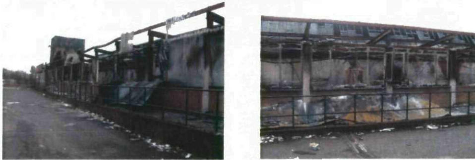
Figure 2.4 – Fire Damage to front elevation of north light block
