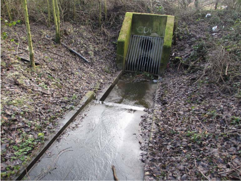
Pipes below Dearne Valley Parkway at end of Spillway
