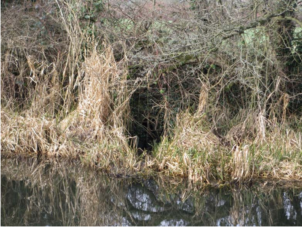
End of 300mm private surface water pipe discharging into canal
