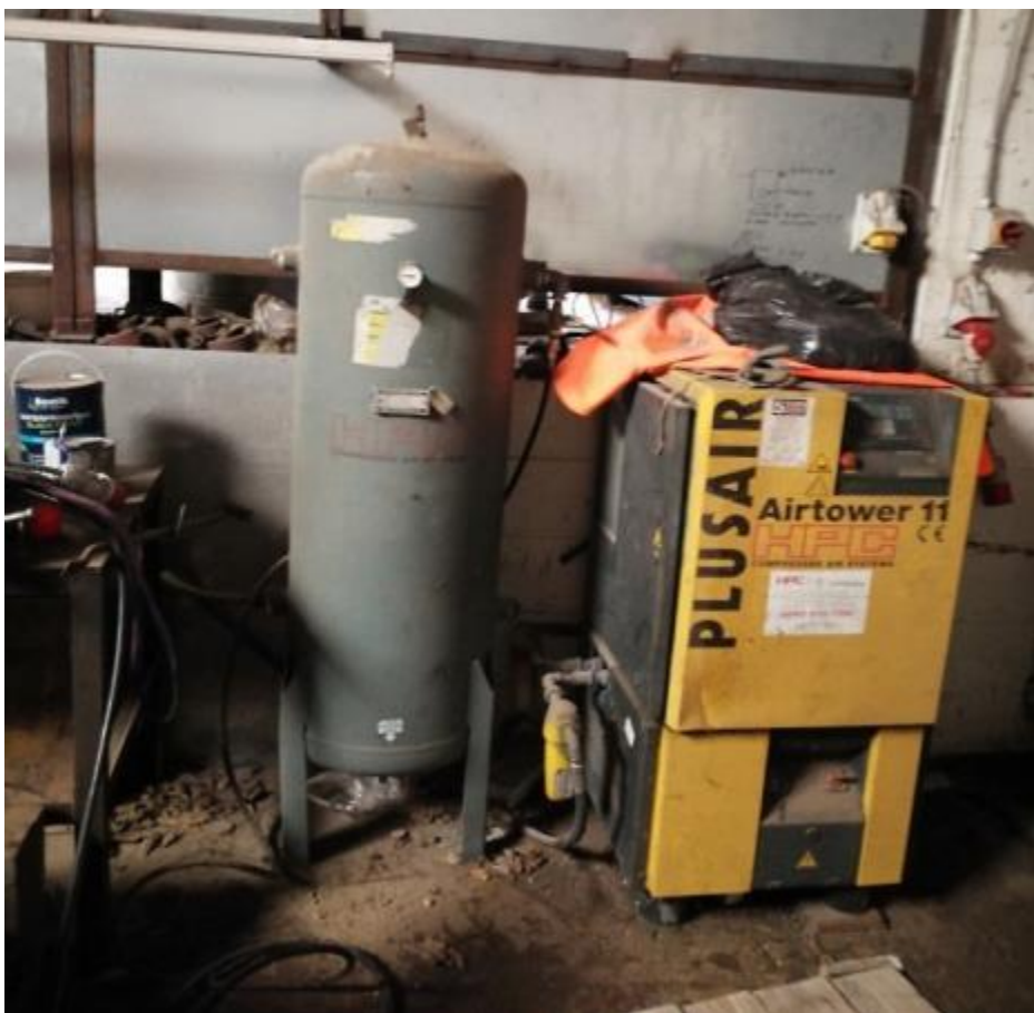
Photograph 12: Compressed air canister inside maintenance workshop
