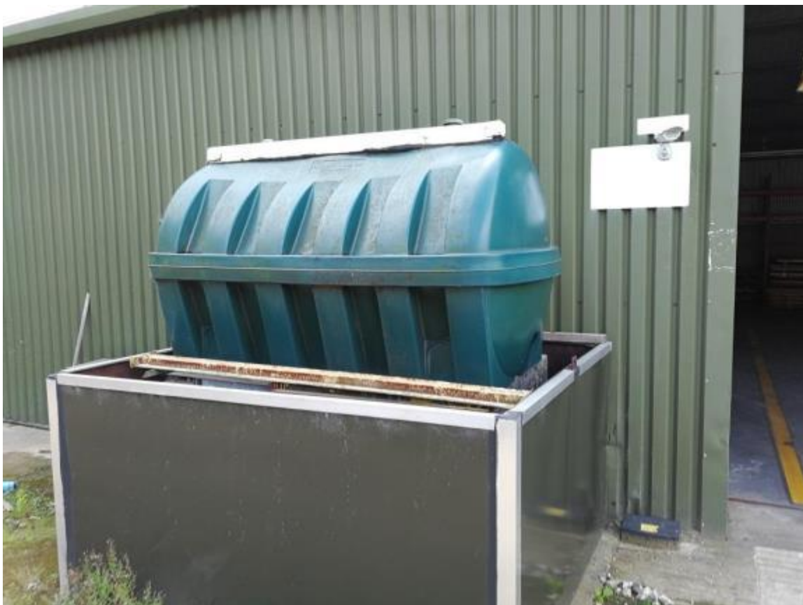
Photograph 34: Bunded above ground diesel storage tank – used for heating
