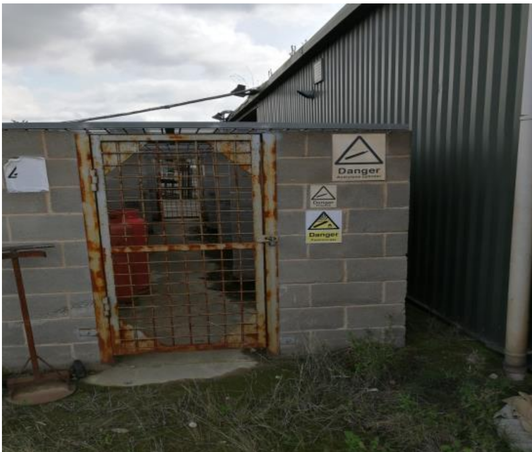
Photograph 20: Secure gas propane gas canister storage area
