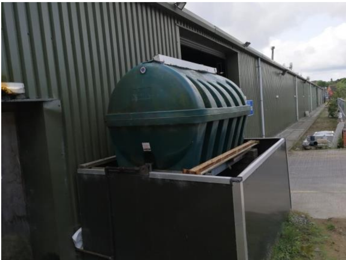
Photograph 36: Diesel storage tank (same as photograph 34)
