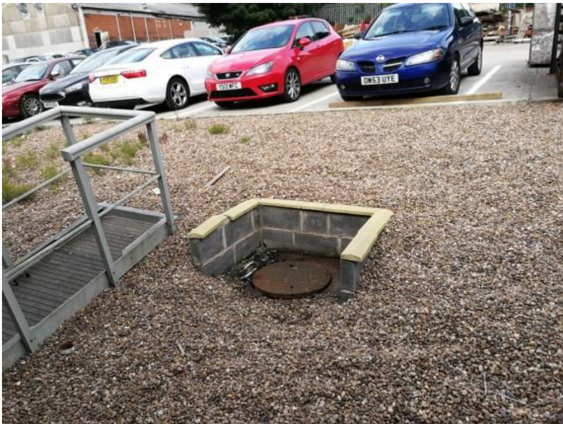
Photograph 43: Manhole for septic tank. According to Bob Irwin pump kicks in when full pumping towards Hough Lane.
