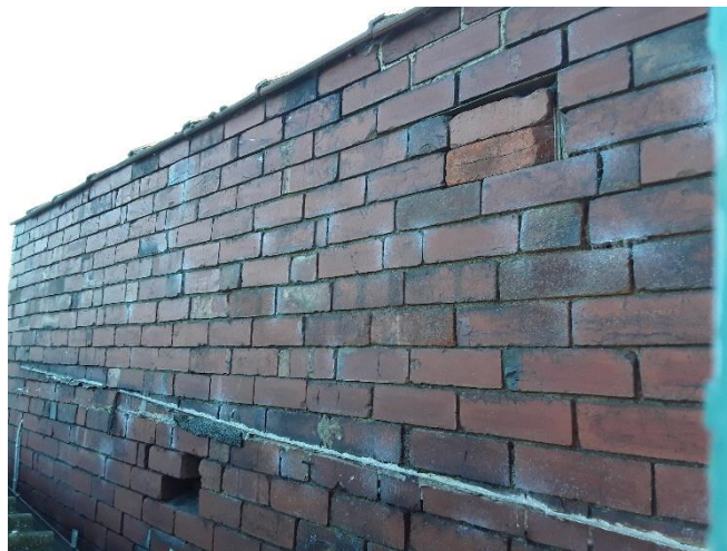
Photograph 2: Loose brick work that may be used as a roost entry point on Building 2
