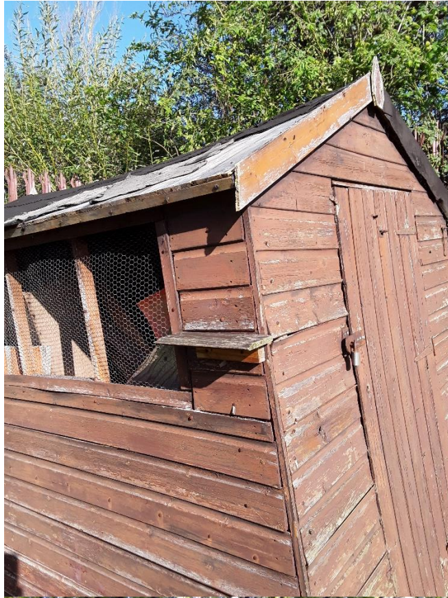
Photograph 4: Torn felt on the roof of Building 4.
