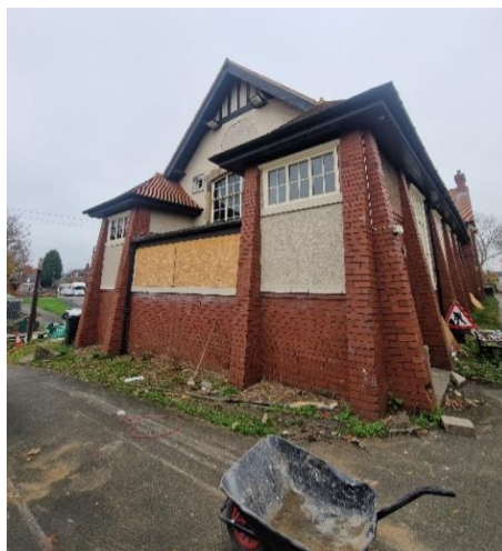
Photo 3. Northwestern elevation of Brierley Village Hall where two hipped-roof columns are present either side of a flat-roofed area. This is the area where the BMS must be adhered to, as detailed below in Section 4.
