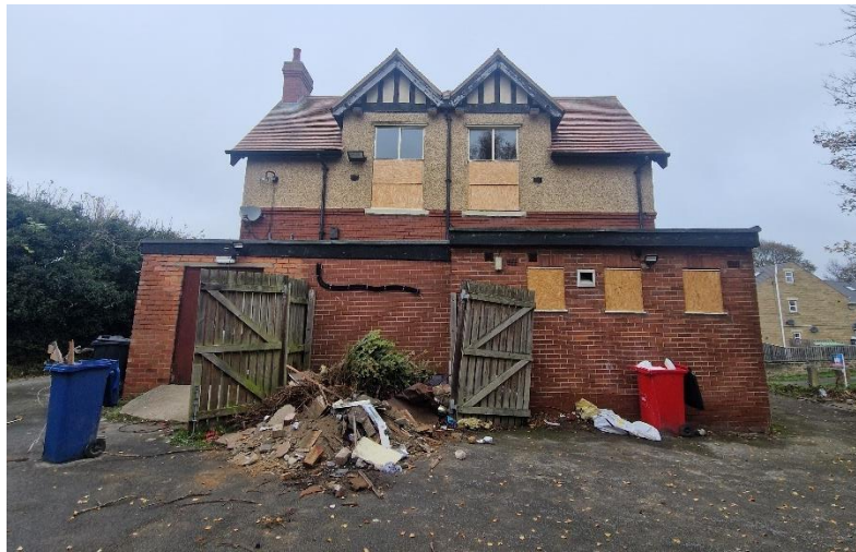
Photo 2. Southeastern elevation of Brierley Village Hall showing the two windows on the first storey that have a small, pitched roof atop, and the one-storey flat roofed extension that is the only section of the building that is to be demolished as part of the Proposed Development.
