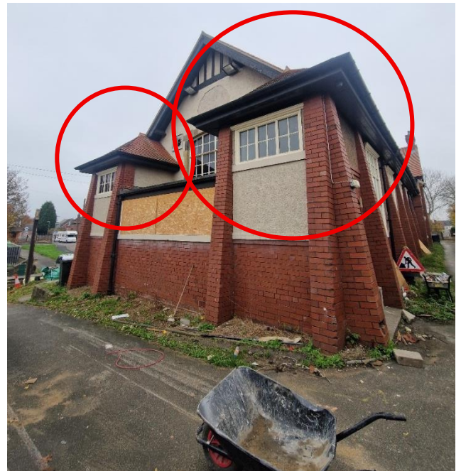
Photo 6. The two areas where internal and external works must be completed April – September (in suitable weather conditions for bats) and supervised by an SQE.
