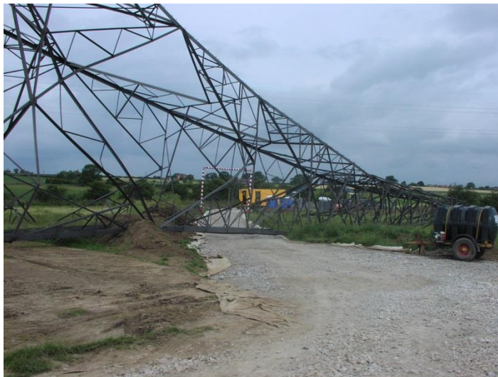
Plate 2.17: Pylon ‘Pulled Over’
