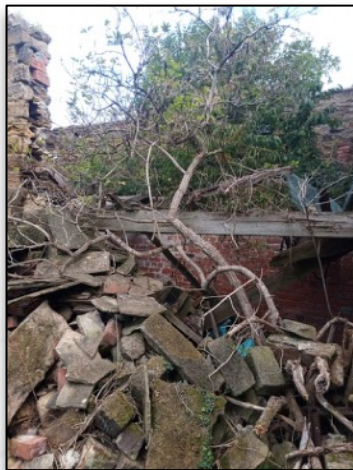
Image 4 - Showing T006, example of poor quality self set tree growing on derelict building edge
