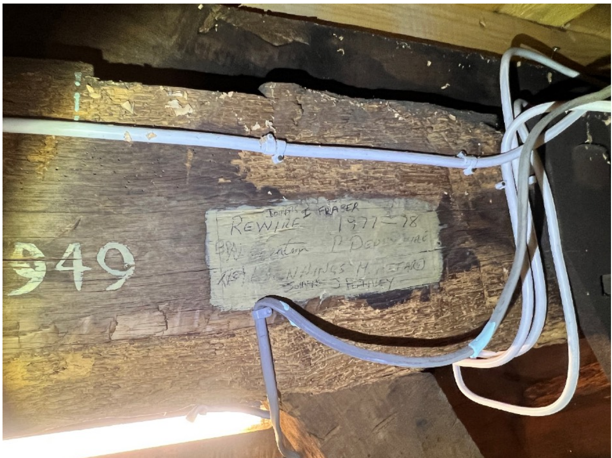
Surface old woodworm to larger section timber to purlins and truss members
