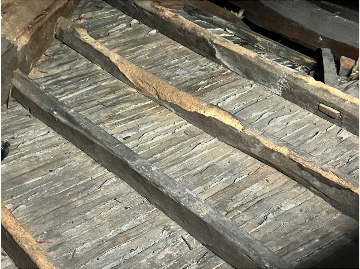
Severely affected ceiling joists above Queen Ann 3
