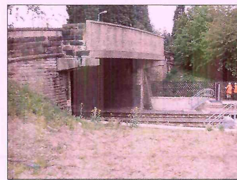
VIEW OF UP PLATFORM, NEAR LOWFIELD ROAD OVERBRIDGE. THIS IS THE PROPOSED PLACE FOR A FOOTBRIDGE
