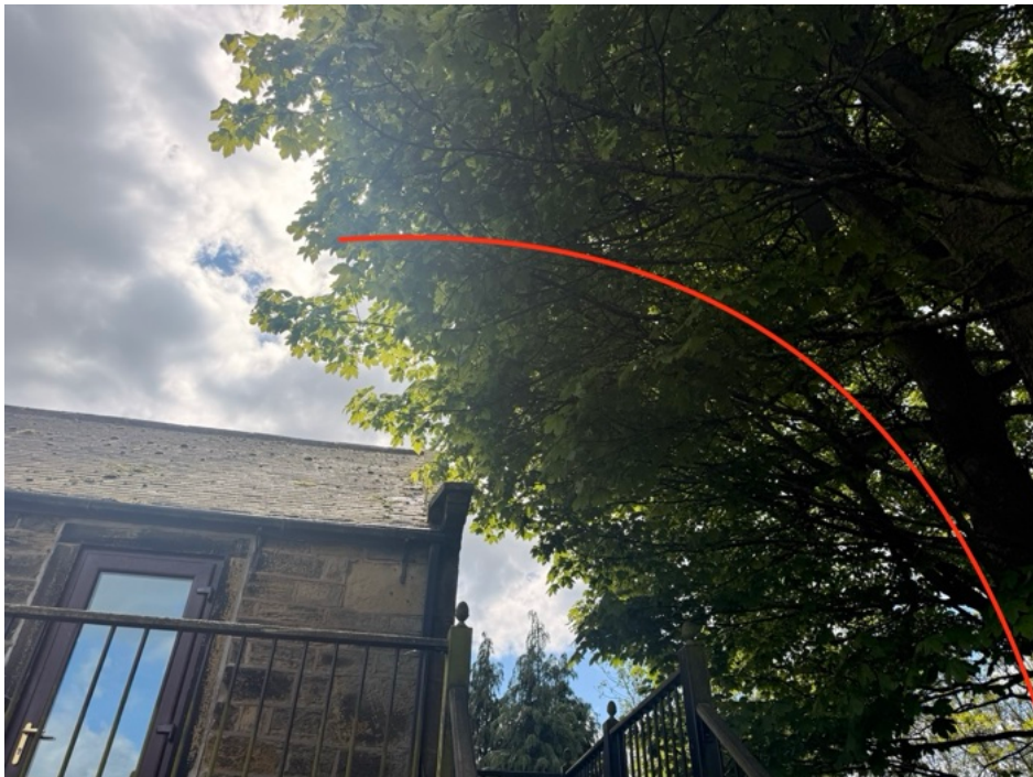
Figure 4. The canopy of T4 is in contact with the building. The red line denotes a potential canopy lift of the eastern aspect of the crown to create a 2m clearance from the building.
