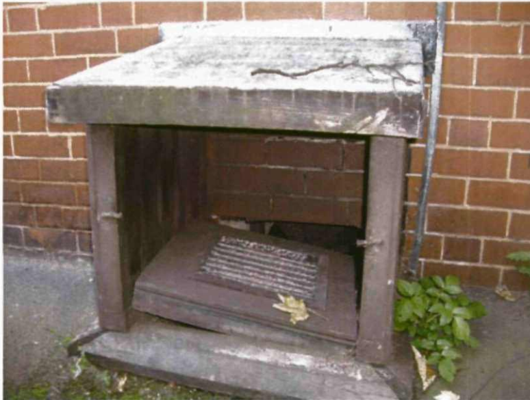
Photo 5: Potential access point for bats, building B1
