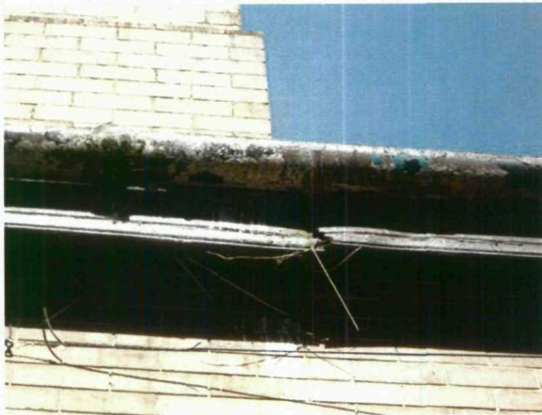
Photo 8: Potential access point for bats, building B4
