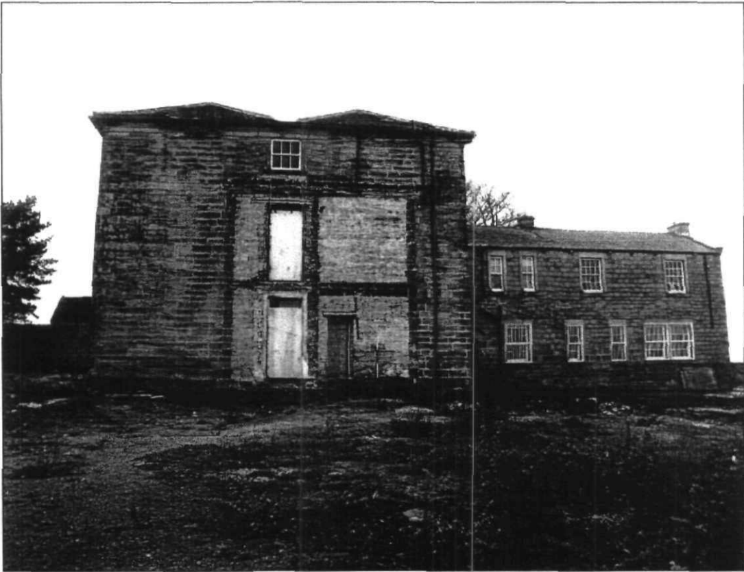
Fig. 28 Southern elevation of Brierley Hall (on the left) and the rear extension (on the right)
