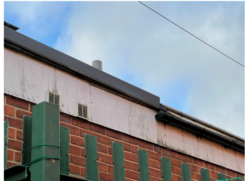
Figure 4 Showing raised tiles on the south-west corner of the building
