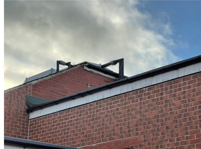
Figure 7 Showing damaged wooden fittings on the north side of the building
