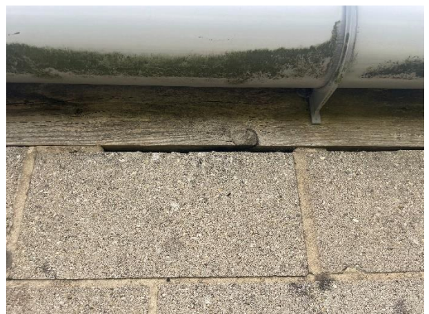
Photo 6: Missing mortar on southern elevation of the building.
