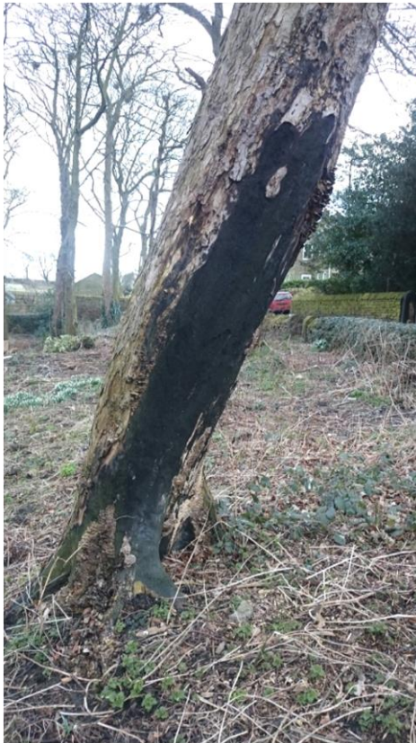
Plate 4. Tree 43, Sycamore. Large area of necrotic bark and wood originating from fire damage. Extensive saprophytic fungi in this area.
