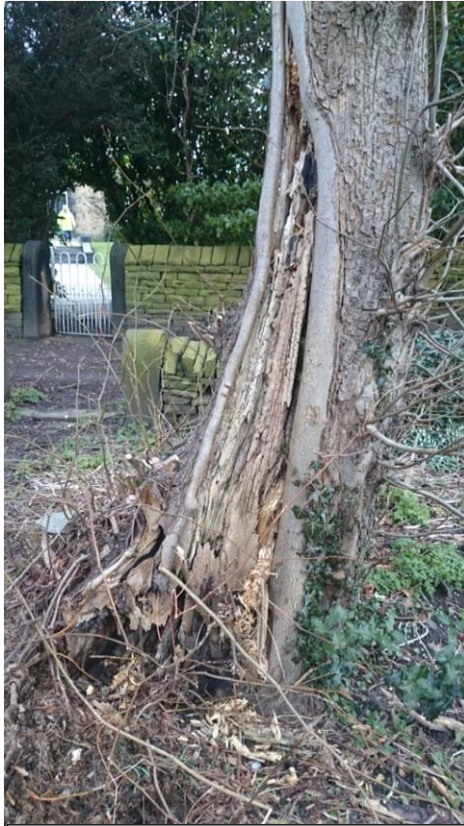
Plate 1. Tree 37, Lime. Stem base severely decayed, on tension side of stem.
