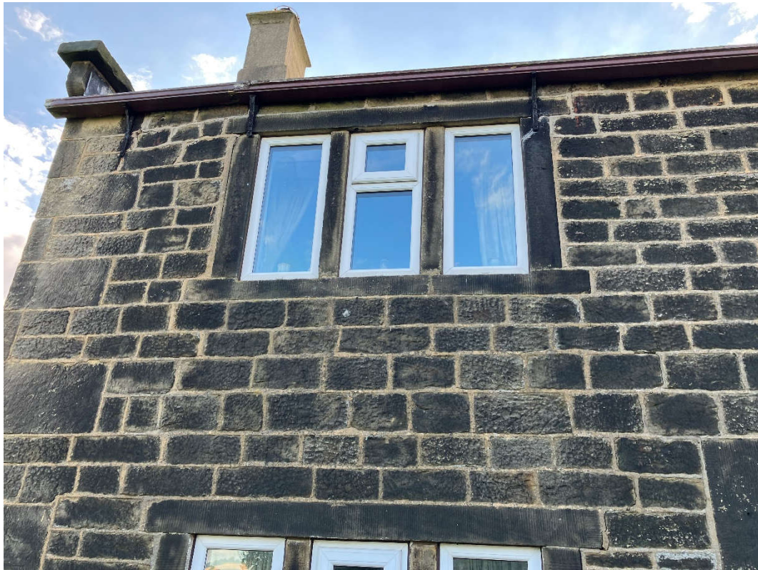
Fig 03. Farmhouse – East first floor window bulging stonework.
