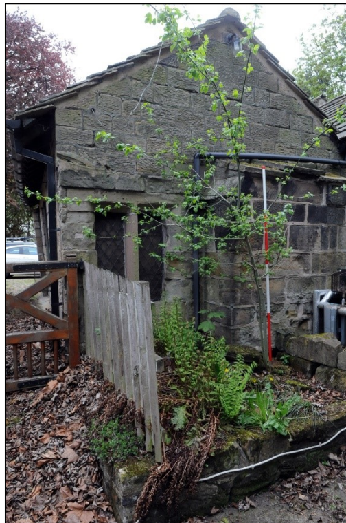
Plate 15: North elevation of Unit 3, including chimney stack and stone mullioned window (Image 120).
