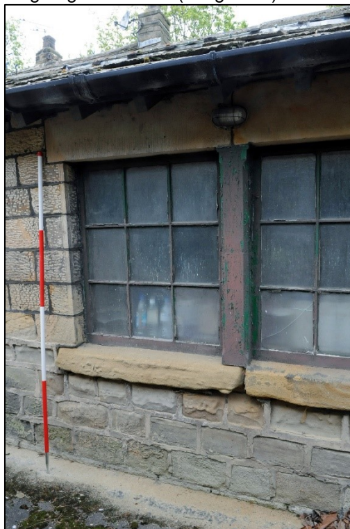
Plate 13: Detail of the window in the eastern elevation of Unit 3, the garage (Image 037).
