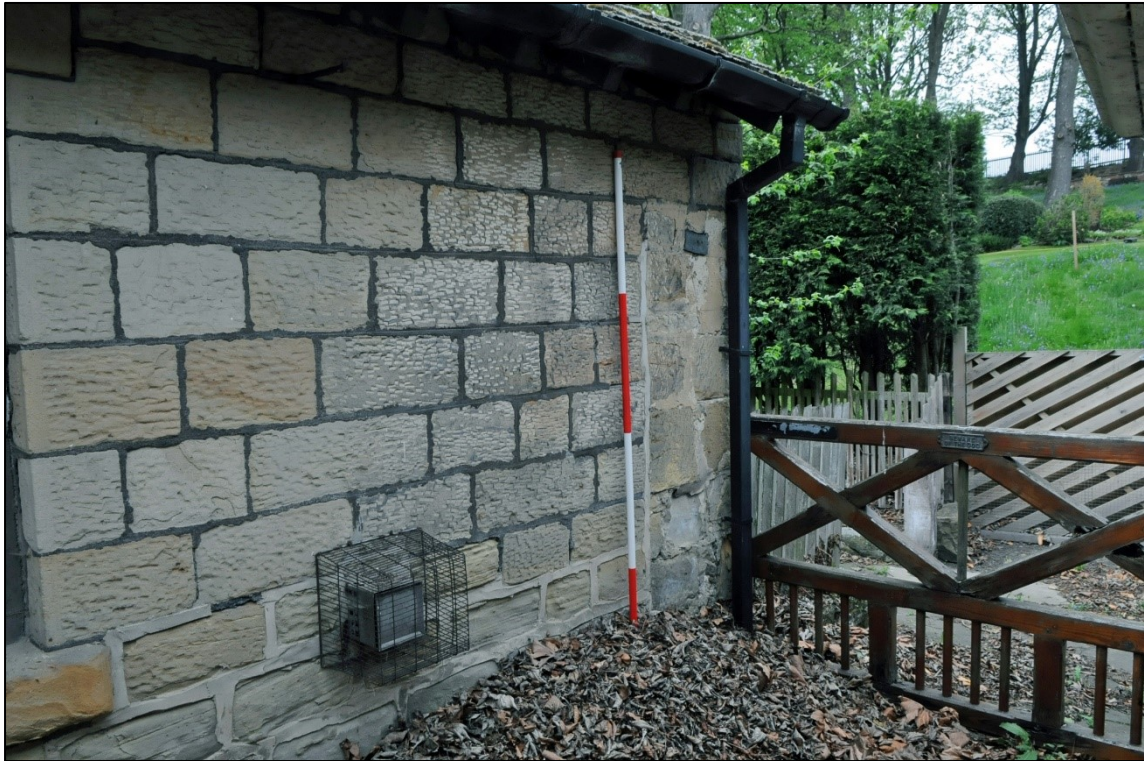
Plate 14: Detail of straight joint in eastern elevation of the 1930s garage extension (Image 036).
