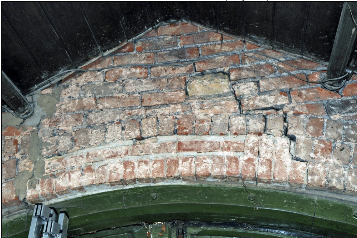
Plate 17: Detail of structural deterioration of the garage building (Image 006).
