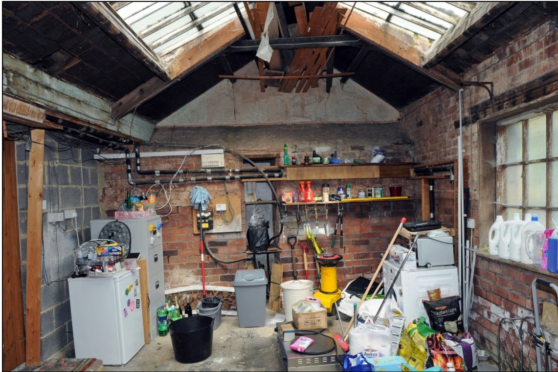
Plate 16: General view of the interior of Unit 3, note brick skin which covers the stone mullioned window, and the blockwork to the left hand side of the frame (Image 001).
