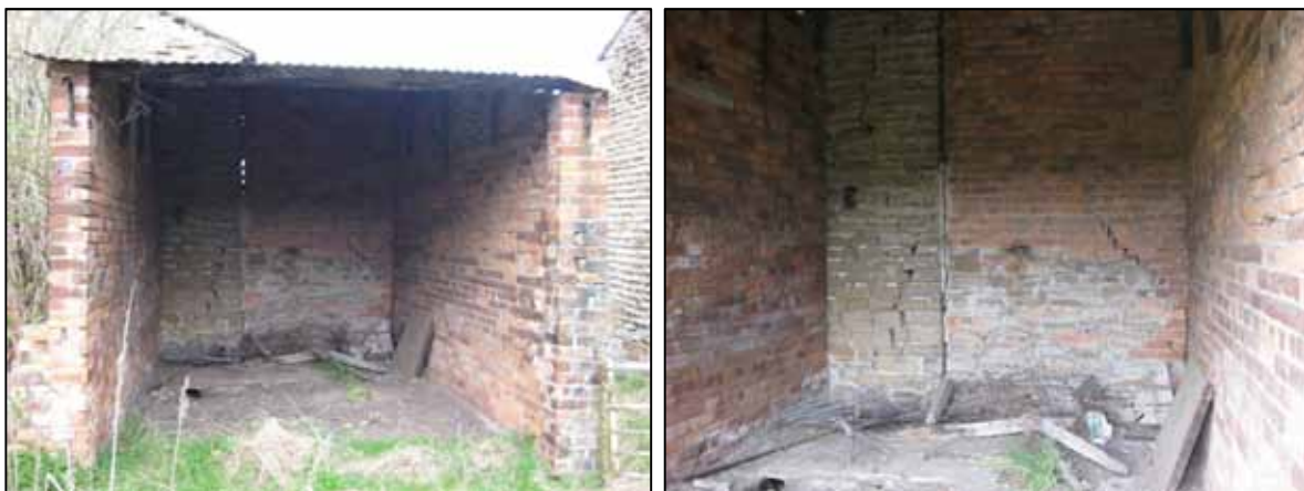
Photographs 42 and 43: Shows a double skin brickwork wall shelter abutting the original coursed sandstone masonry construction, built off of the existing ground which is inadequate founding material without proper footings etc. Spare pieces of timber have been used to act as purlins to support a corrugated roof. Cracking in both the brickwork and coursed sandstone is evident. A line of mortar is the only restraint fixing currently visible between the old and new construction. As such it is our opinion that this area be taken down and rebuilt with adequate fixings and adequate foundations.
