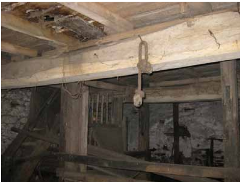
Photograph 78: Illustrates the first floor layout in the Agricultural 'Building B'. The first floor comprises of oak supporting beams, with softwood joists. The timber floor planks show signs of decay, and should be replaced where necessary
