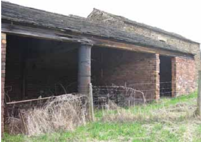
Photograph 64: Illustrates the west elevation of the Agricultural Building 'B'. The majority of this area is newer brickwork, which is in good condition. However the supporting eaves members are decayed and would require replacing. The cast iron stanchion is used as a column to support the timber roof, and if kept would demonstrate the diversity of building materials used in the past. The adequacy of the foundations in this area may require investigating.
