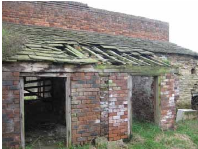
Photograph 59: Details the condition of the roof and existing brickwork walls to the end of the East Elevation. This area is adjoining the main coursed sandstone masonry building. It is evident that the buildings have been added to over the years due to the number of different brick types used as well as the different mortar. The roof members should be discarded as the roof is in a state of disrepair. The tying of each of the sections of the walls looks to be insufficient which would account for the signs of movement and the voids between the different wall types.
