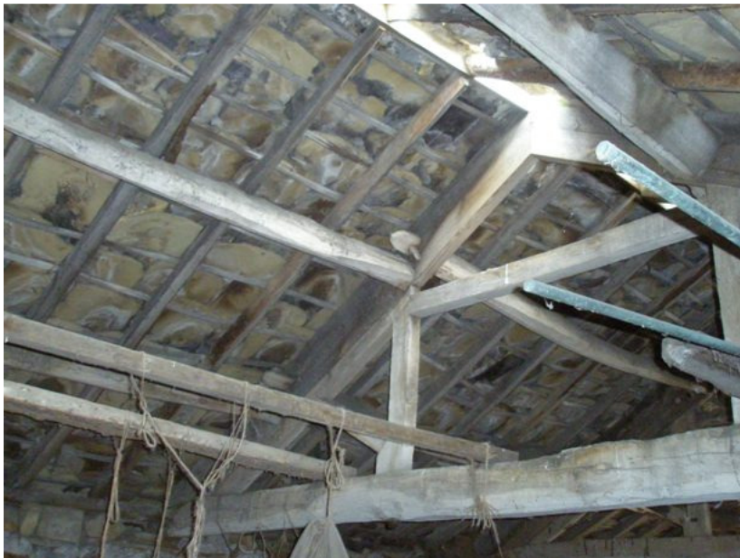
Photograph 83: Shows the timber roof truss layout in the Agricultural 'Building 'B'. The truss appears to be a mixture of oak and softwood. All the timber elements look aesthetically in a good condition, but further assessment may be required due to their age.
