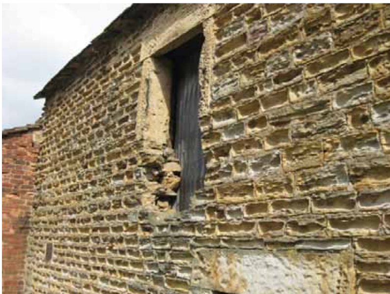
Photograph 74: Shows the West elevation, and the area needing repair around the first floor opening. Deterioration of the coursed sandstone masonry is again evident. We would estimate that 5% of the coursed sandstone could be reused from this elevation.
