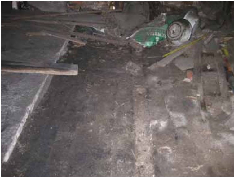
Photograph 77: Shows the construction of the ground floors within the building. To the right of the photo shows the cobbled floor with a concrete slab to the left.
