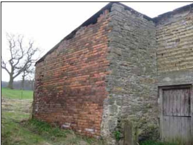
Photograph 46: Shows the North-east elevation, and demonstrates the connection between old and new construction. There is considerable cracking towards the bottom of the sandstone masonry and there is also signs of movement as the sandstone masonry deviates from horizontal.
