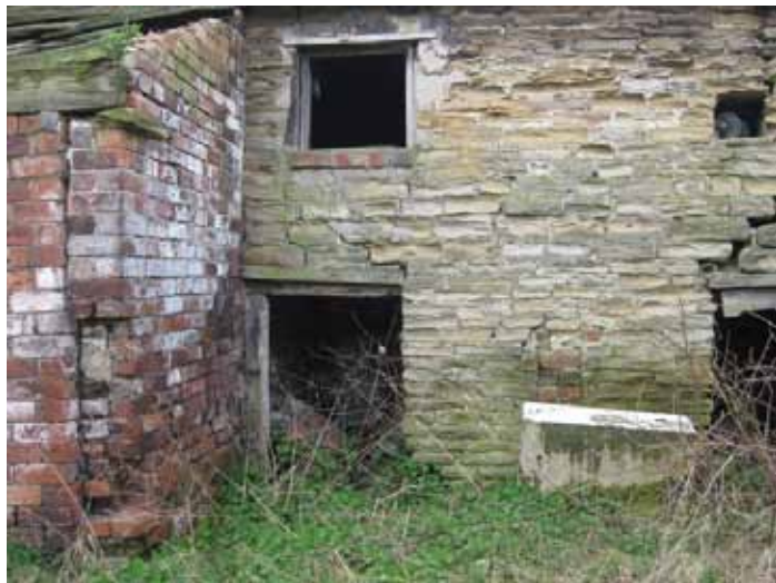
Photograph 61: Shows signs of movement with the lintels and masonry deviating from horizontal. The tying of each of the wall sections looks to be inadequate which would account for the signs of movement and the voids between the different wall types. There are several voids above the lintels, 80mm in width; however the coursed sandstone masonry looks to be in a comparatively good condition. Most of the masonry units could be reused.
