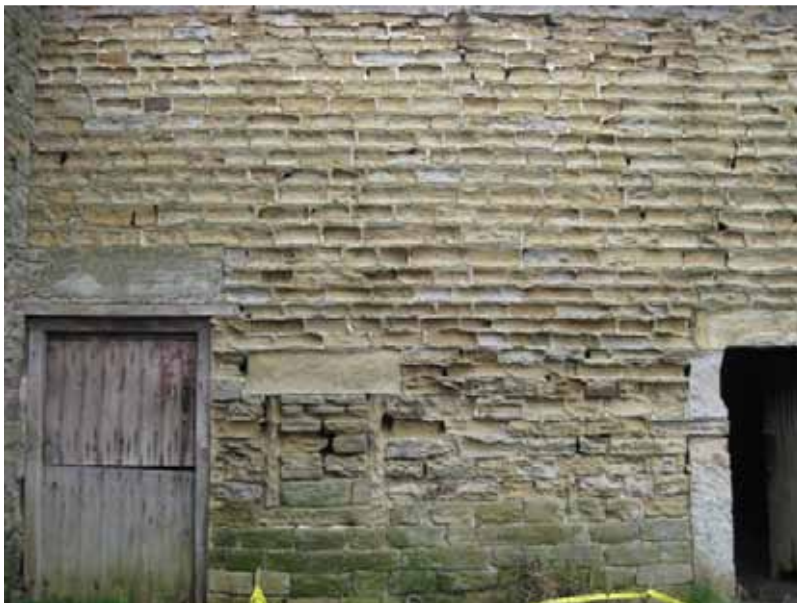
Photograph 50: Shows the East elevation. There are many voids present, as well as cracking and signs of movement. Deteriorations of the coursed sandstone masonry is also evident with areas of absent mortar.
