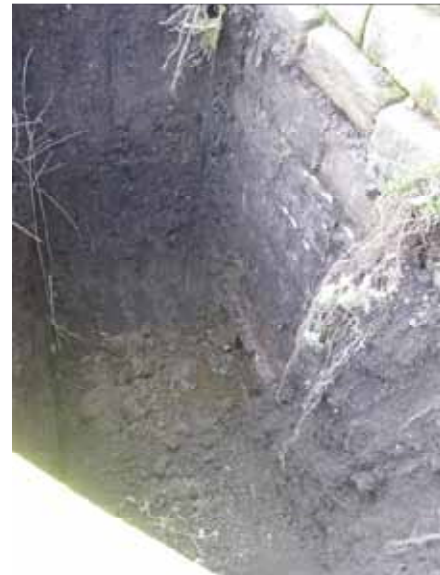
Photographs 4 and 5: Details the trial hole at the East elevation. The trial hole is 1.6m in depth and shows the existing foundations at this depth. The ground is made up of top soil to approximately 1.6m, with signs of stiff clay beneath. The foundations appear to be adequate in their current state, and would not need to be replaced.
