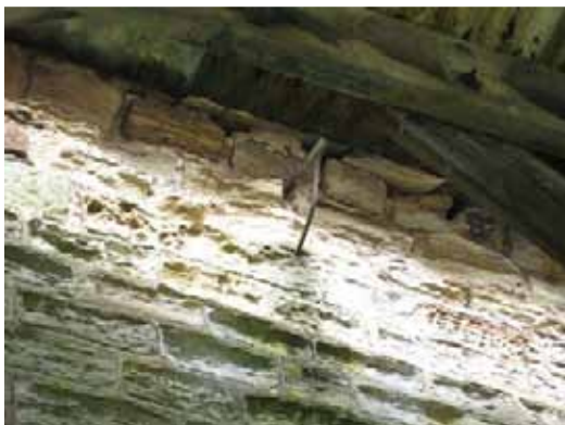
Photograph 29: Shows eaves level at the rear of the property (South elevation). There is evidence of frost damage to the high level sandstone masonry and mortar, with visible voids between the stonework.
