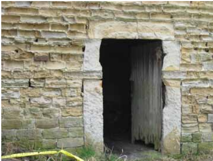
Photograph 54: Shows the East elevation. The lintel over the opening shown has significant cracks, which may be from movement rather than buckling. There are many voids present, as well as cracking and signs of movement in the masonry. Deteriorations of the coursed sandstone masonry is also evident with areas of absent mortar.
