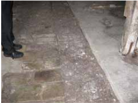
Photograph 38: Shows the construction of the ground floors within the building. To the left of the photo shows cobbles with a central drain run, with a concrete slab to the right.
