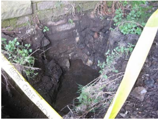
Photograph 23: Details the trial hole at the South elevation. The trial hole is 1.0m in depth and shows the existing foundations at this depth. The ground is made up of top soil to approximately 1.0m, with signs of stiff clay beneath. The foundations appear to be adequate in their current state.
