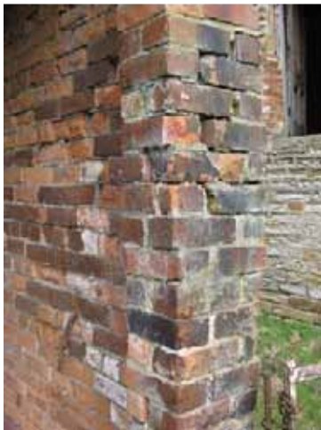
Photograph 45: Shows the brickwork masonry pier with considerable cracks and loose bricks. Again it is our opinion that this area be taken down and rebuilt with adequate fixings and adequate foundations.
