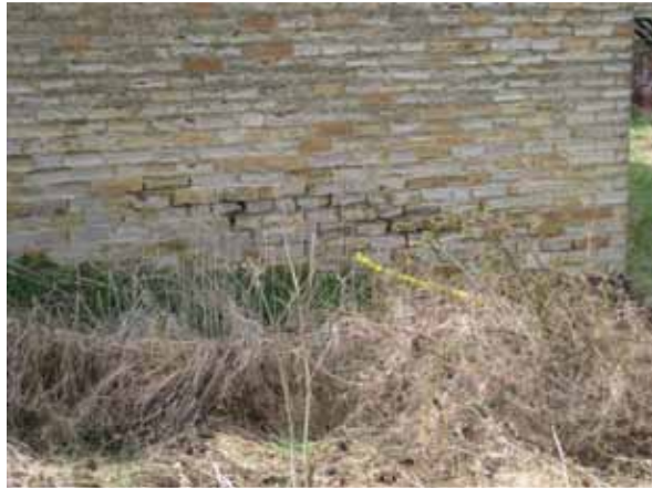
Photograph 32: Illustrates the extent of the open joints in the East elevation wall at low level. However this is only due to the absence of mortar between the coursed sandstone masonry
