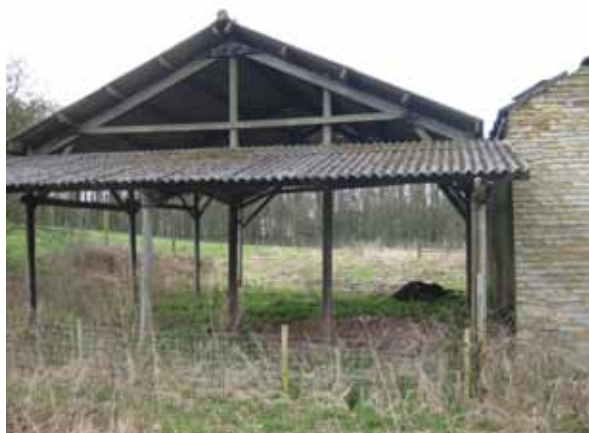
Photograph 34: Shows the side structure adjoining Agricultural Building 'A'. It consists of timber posts, haunches and trusses with a corrugated roof. It has no major defects, but would serve no purpose for conversion to alternative use, and should therefore be removed.
