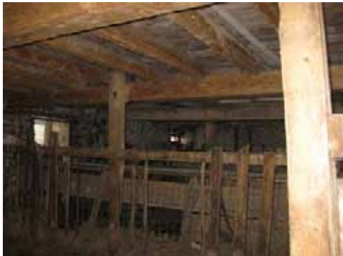
Photograph 39: Details the layout of the underside of first floor. The timber supporting beams and columns are softwood and are generally in a good condition; however the floor boards have aged and are decayed in some areas.
