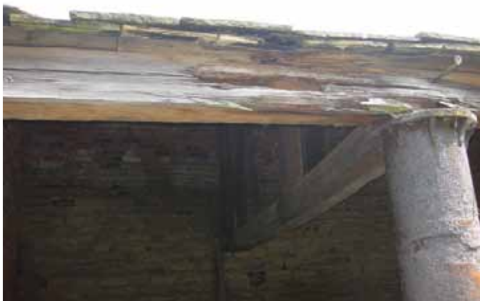
Photograph 65: Shows the eaves members to the west elevation supported by the cast iron haunch. It can be clearly seen that the eaves timber is decayed and would need to be replaced.
