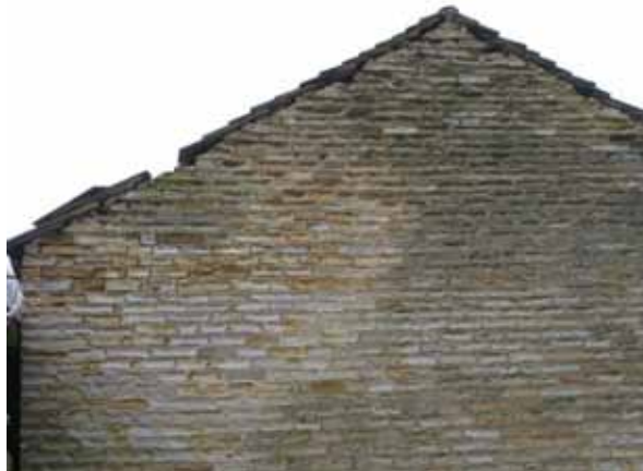
Photograph 33: Shows the slate roof over the East elevation gable. Frost erosion may have caused the mortar to deteriorate and roof slates to become loose.
