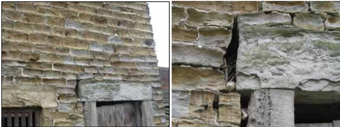
Photographs 55 and 56: Shows the end doorway on the East elevation. The movement in the building has resulted in 80mm cracks/voids being formed in the masonry. The existing lintels could be reused.
