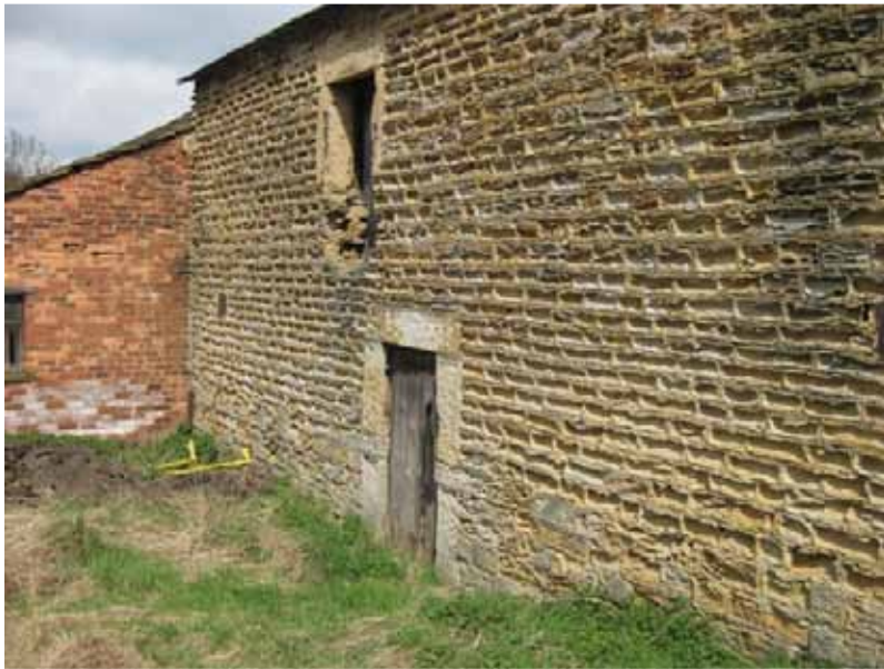
Photograph 72: Shows the West elevation and the extent of the soil migration of the years, culminating in the external levels immediately in the vicinity of the doorway being higher than the internal finished floor level. There are many voids present, deteriorations of the coursed sandstone masonry is also evident.
