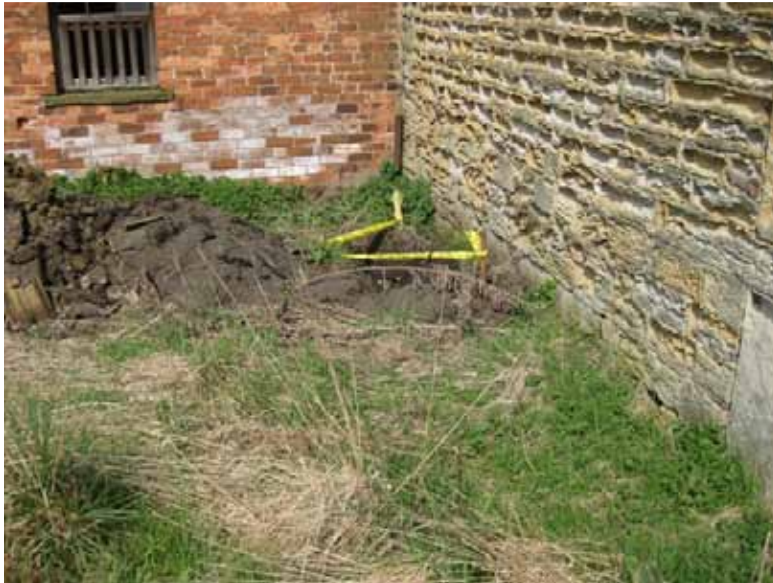
Photograph 75: Shows the West elevation and the extent of the soil migration of the years, culminating in the external levels being higher than the internal finished floor level. The soil characteristics are top soil down to 1m deep, with firm to stiff clay below.
