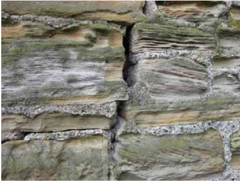
Photograph 48: Shows a 45mm crack in the North-east elevation, as described above in Photograph 46. There has been significant movement and therefore may suggest subsidence or inadequate foundations.
