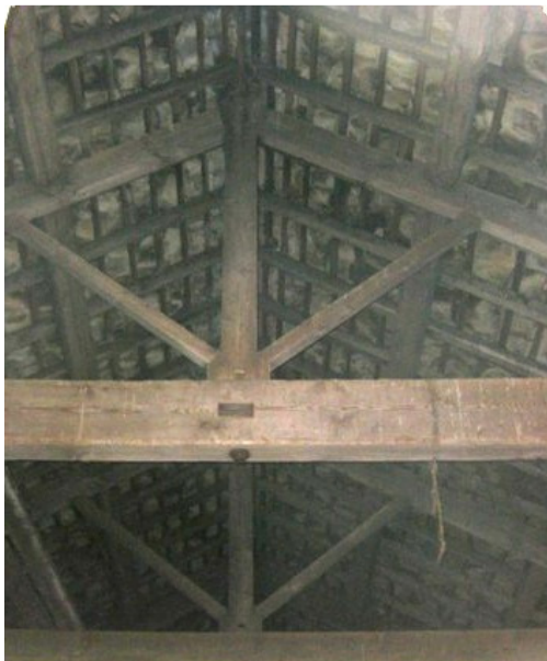
Photograph 40: Shows the layout of the softwood roof structure; King Post truss with purlins and rafters. These all look to be salvageable and it is our opinion that these could be re-used where possible.
