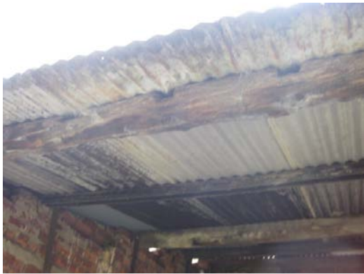
Photograph 44: Shows the timber pieces currently used as purlins to support the corrugated roof on the south elevation. The timber pieces are significantly decayed and should be discarded.
