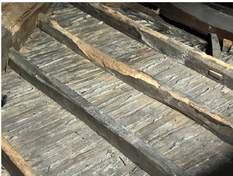
Photo showing the reduced size of timbers. New timbers of similar size will be placed alongside and screwed to the existing.
