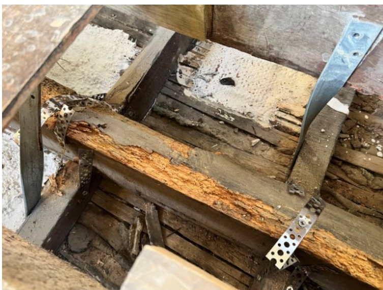
Similar damage has occurred in the floor void below the south of the long gallery.
