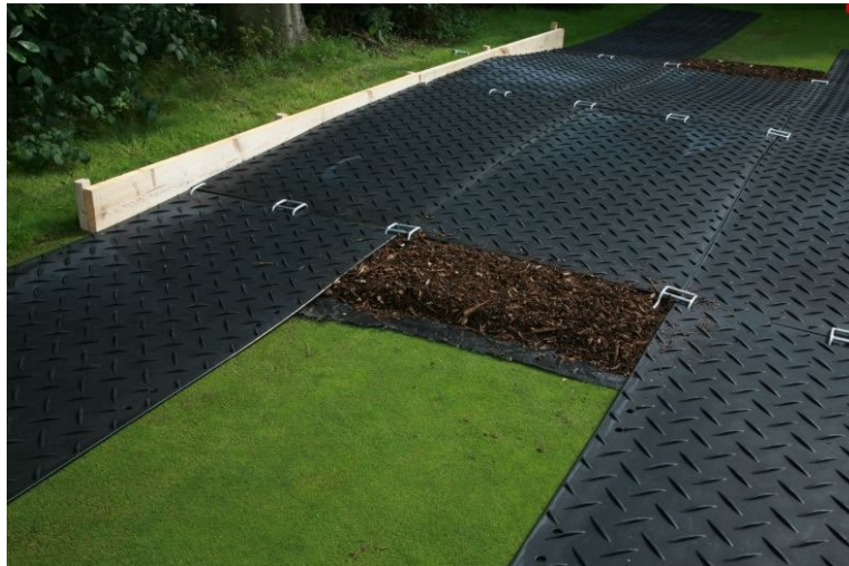
Figure 4. Ground protection interlinked plastic boards with a layer of wood chippings at least 150mm deep.
