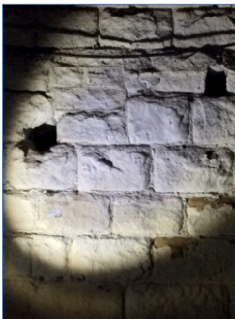
Photograph 34. Internal view of some of the gaps in stonework of B10 (TN11)
