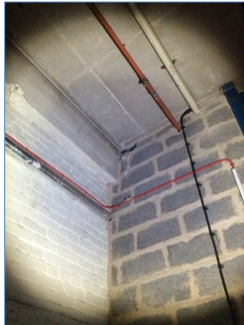
Photograph 27. Internal view of ground floor B23 - typical brick, breeze-block and concrete construction
