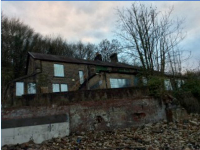
Photograph 30. Subterranean external wall of a demolished building (TN17), adjacent to B18 (seen beyond)
