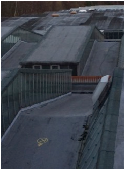
Photograph 26. Pre-fabricated steel roofing showing window system – B21, viewed from 2 nd floor B22
