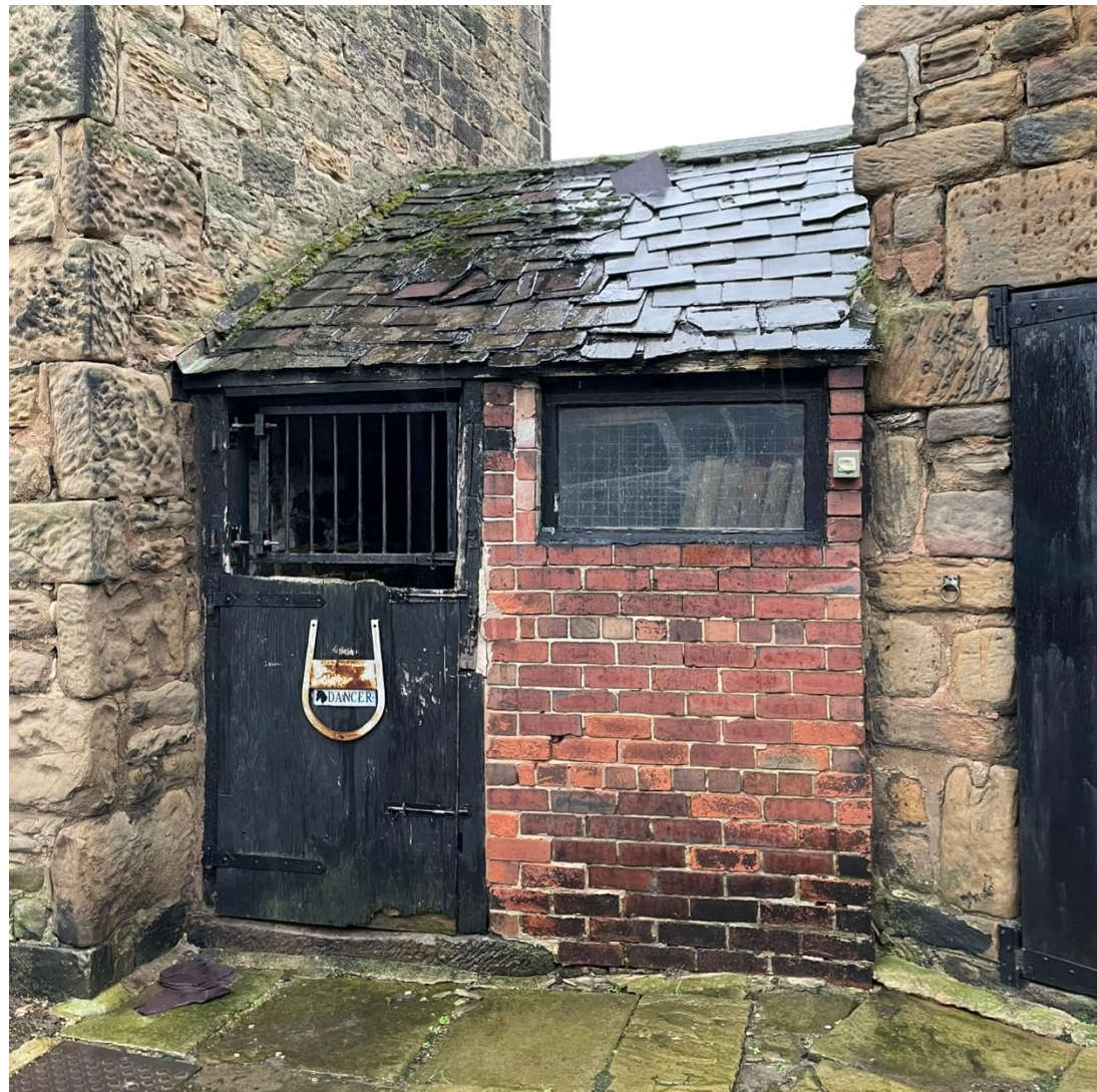
Figure 10 View of west elevation of The Stable, with slate half of the roof visible.
