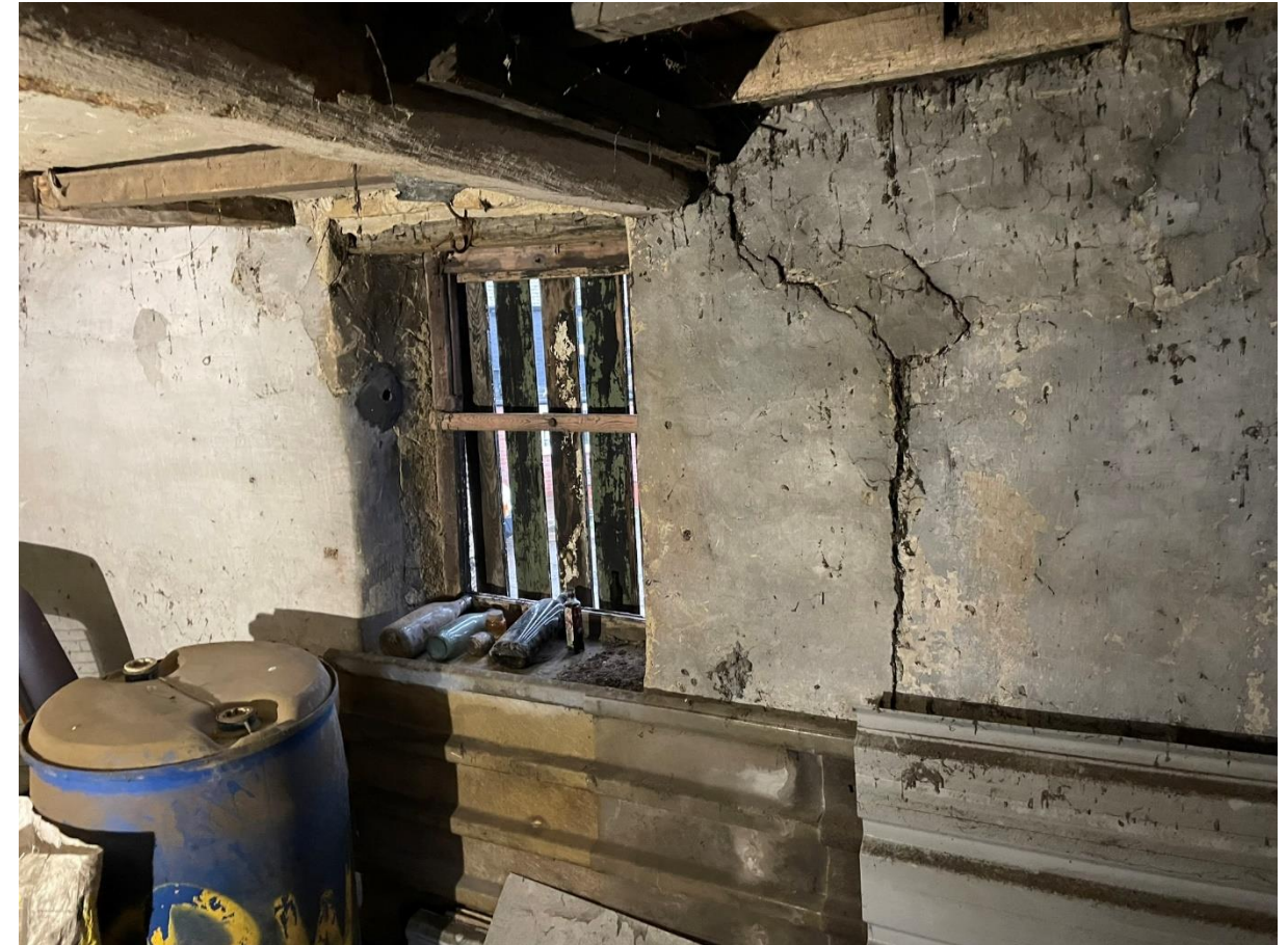
Figure 16 Crack in plaster at first floor level adjacent to window on west elevation corresponding with partial infill of window.
