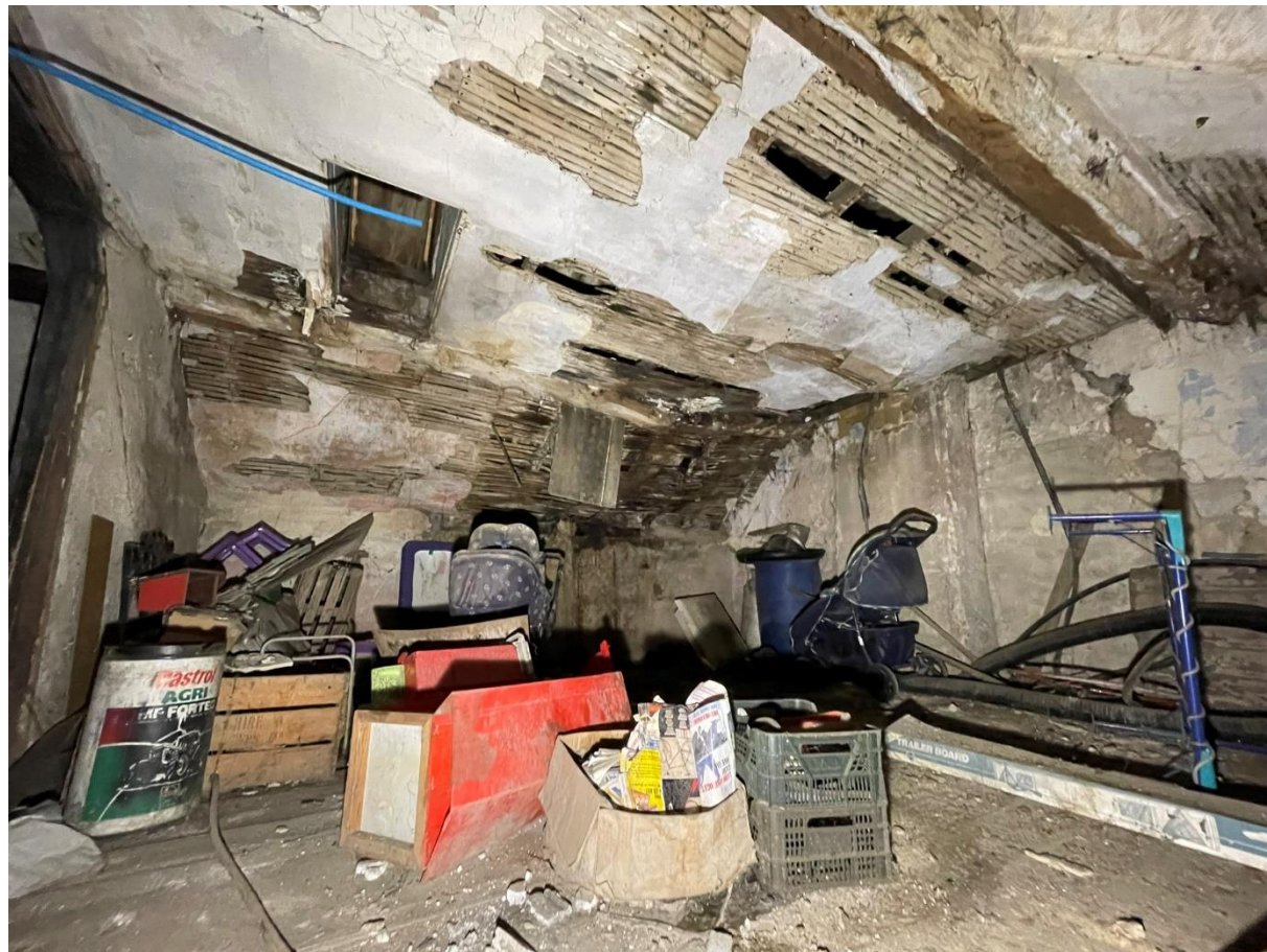
Figure 12 Failure of purlin visible to rear of image.
