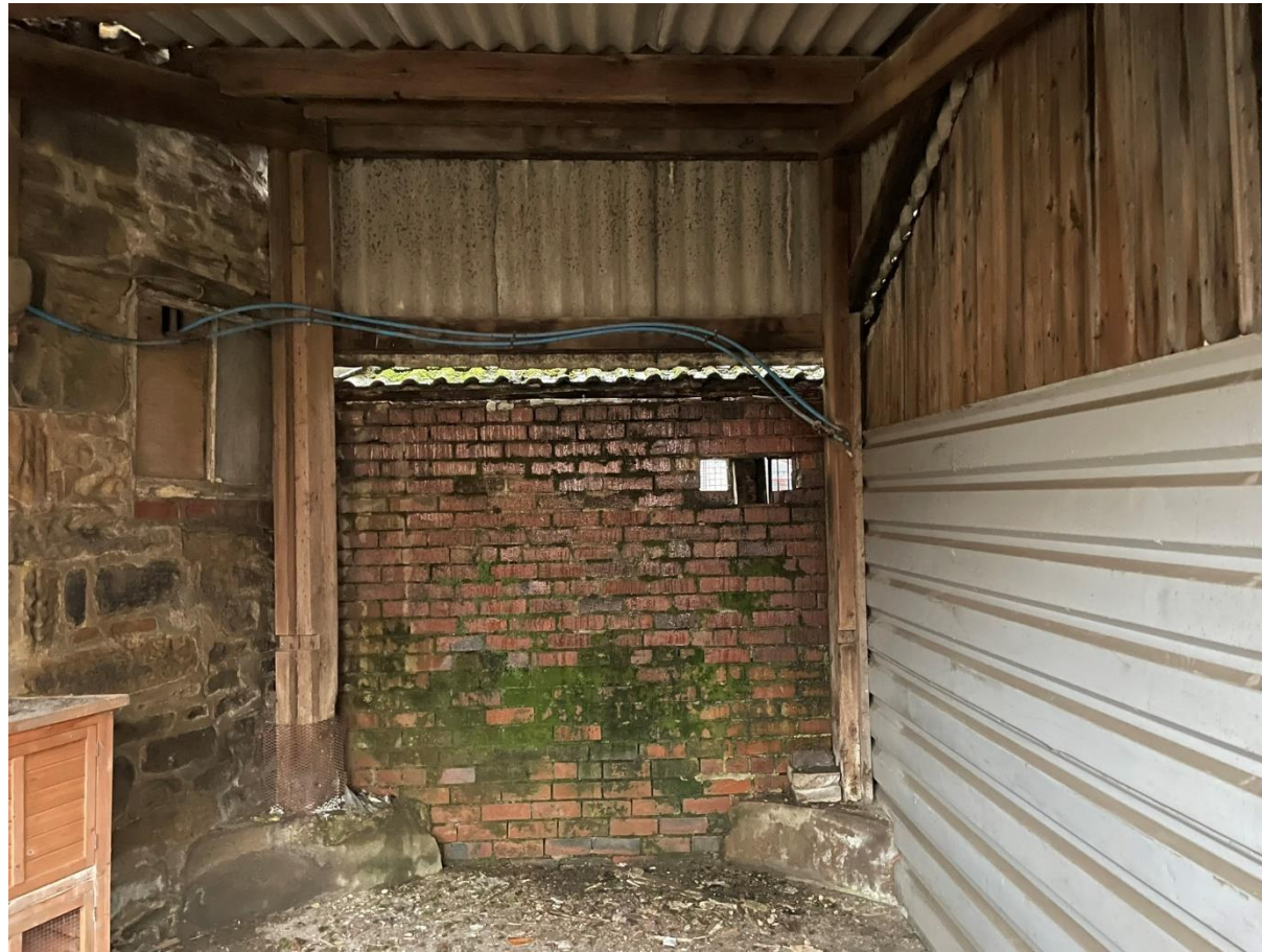
Figure 19 East elevation of The Stable with brickwork missing from external wall.
