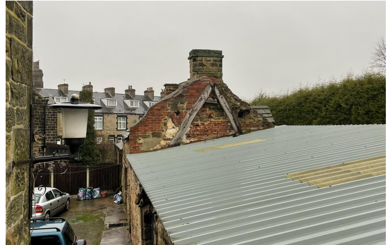
Figure 5 The Cottage eastern gable. Cruck frame from the agricultural store visible projecting through the roof against eastern gable of The Cottage.
