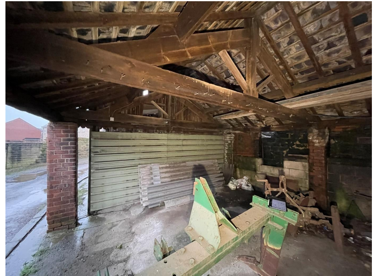
Figure 9 Internal view of covered area of The Corn Chamber. Brick piers visible supporting king post trusses, with corrugated sheeting and timber panel partition to background.
