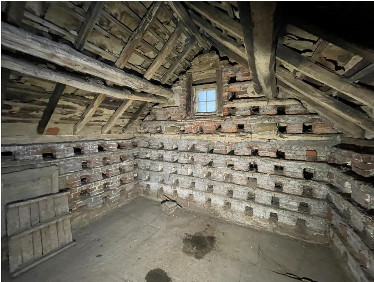
Figure 8 Second floor of main building of The Corn Chamber with stone flags visible.
