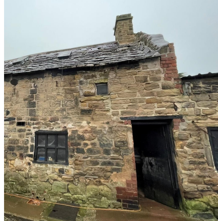
Figure 11 Cement-based mortar, brickwork repairs, and brick gable all visible to south elevation of The Cottage.
