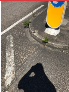
ISSUE 14 DAMAGED KERBS TO THE CROSSING POINT TO THE RETAIL UNITD
