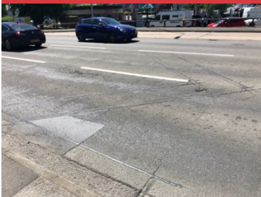
ISSUE 35 DAMAGED TARMAC ADJACENT TO TESCO PFS
