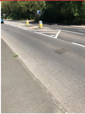
ISSUE 21 DAMAGED MANHOLES IN WOMBWELL RD
