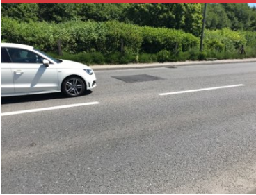
ISSUE 2 HIGHWAY TARMAC REPAIRS LIFTING
