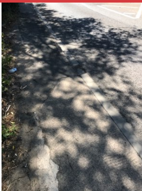
ISSUE 27 DAMAGED KERBS ADJACENT TO HARVEY S
