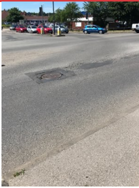
ISSUE 33 DAMAGED TARMAC AROUND MANHOLES ADJACENT TO TESCO BELL MOUTH
