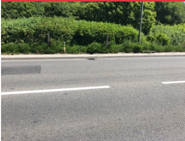
ISSUE 3 HIGHWAYS DAMAGED DRAIN COVER
