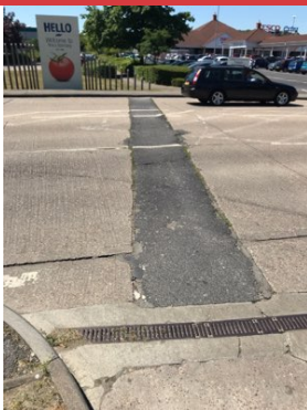
ISSUE 11 DAMAGED TARMAC STRIP LEAVING TESCO PFS
