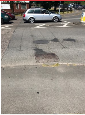
ISSUE 17 DAMAGED TARMAC GOING INTO THE TESCO CARPARK A
