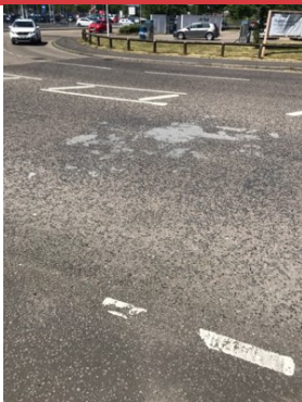
ISSUE 16 DAMAGED TARMAC GOING INTO THE TESCO/RETAIL BELL MOUTH
