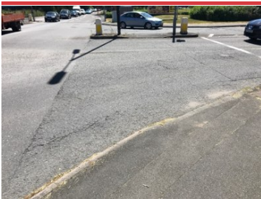
ISSUE 8 TARMAC DAMAGE IN LEFT HAND LANE LEAVING TESCO
