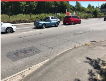
ISSUE 6 TARMAC DAMAGED TURNING LEFT FROM TESCO
