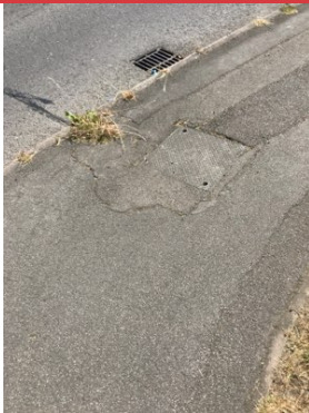
ISSUE 7 FOOT PATH DAMAGE AROUND COVER
