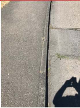
ISSUE 13 DAMAGED KERB NEXT TO THE TESCO HELLO WALL
