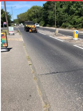
ISSUE 24 CRACKED TARMAC ADJACENT TO SUBWAY
