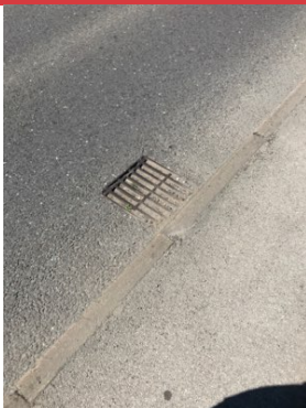
ISSUE 32 BLOCKED GULLIES ADJACENT TO TESCO BELL MOUTH
