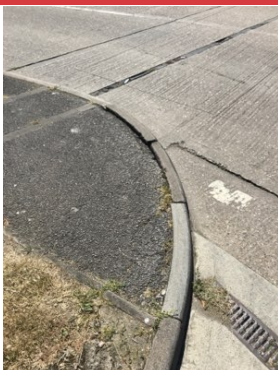
ISSUE 12 DAMAGED KERBS LEAVING TESCO PFS
