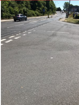
ISSUE 22 CRACKED TARMAC IN B&M BELL MOUTH
