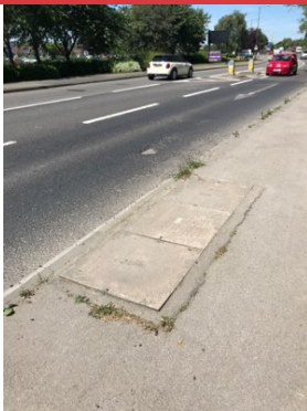
ISSUE 26 DAMAGED BT COVERS
