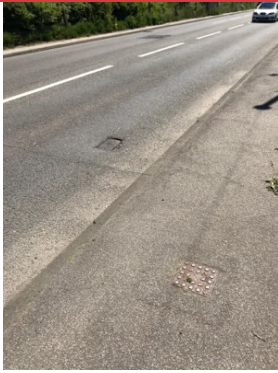
ISSUE 1 DAMAGED WATER HYDRANT
