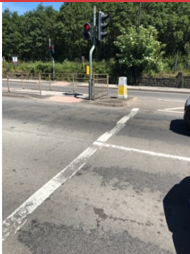
ISSUE 19 DAMAGED KERBS ON THE ISLAND ON THE WOMBWELL RD
