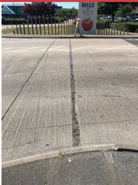
ISSUE 10 DAMAGED BOUNDARY MARKERS LEAVING TESCO PFS
