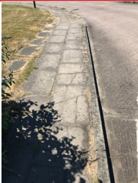
ISSUE 15 CRACKED SLABS LEFT HAND SIDE GOING INTO THE RETAIL PARK
