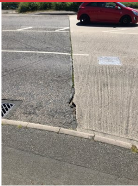
ISSUE 9 DAMAGED TARMAC NEXT TO CONCRETE TESCO CONCRETE BOUNDARY
