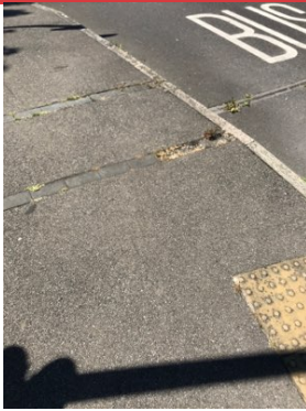
ISSUE 5 BLOCK PAVING DAMAGED IN THE BUS LANE FOOT PATH
