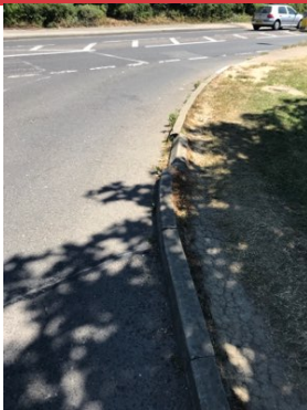
ISSUE 23 DAMAGED KERBS IN B&M BELL MOUTH
