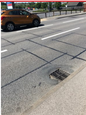
ISSUE 36 DAMAGED GULLY ADJACENT TO THE TESCO BUS LANE
