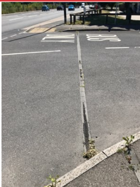
ISSUE 4 ACO DAMAGED IN THE BUS LANE
