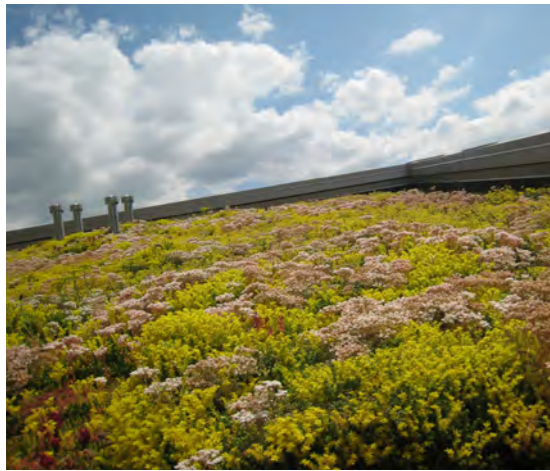
Intensive green roof
