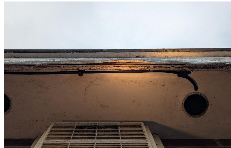
Figure 5 View of gap in soffit box.
