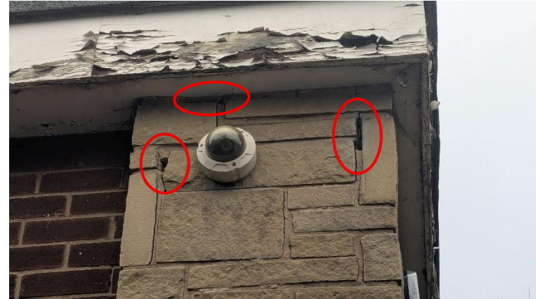
Figure 4 View of gaps in the stone pillar.
