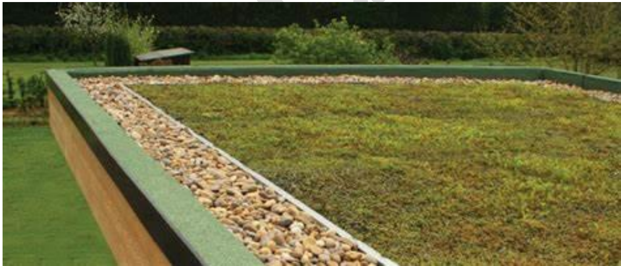
Example of simple green sedum roof
