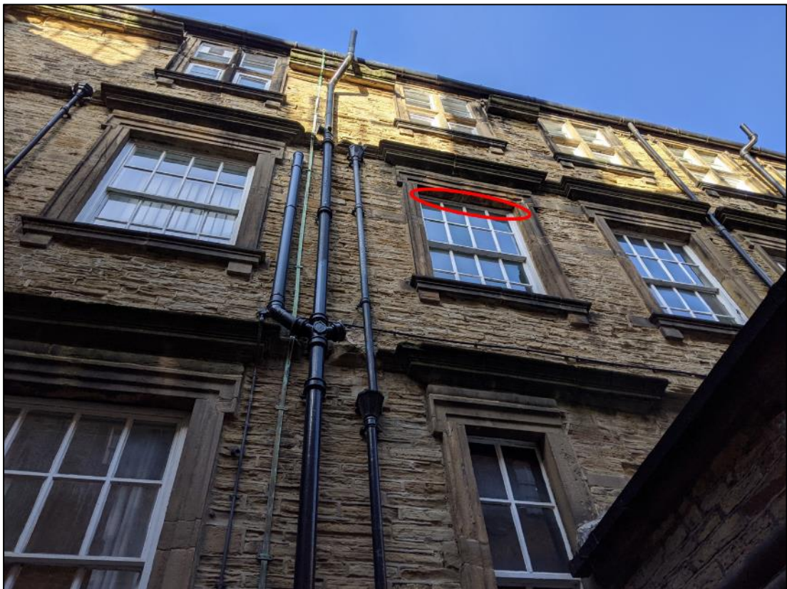
Plate 8. Crevice between damaged lintel and frame within courtyard
