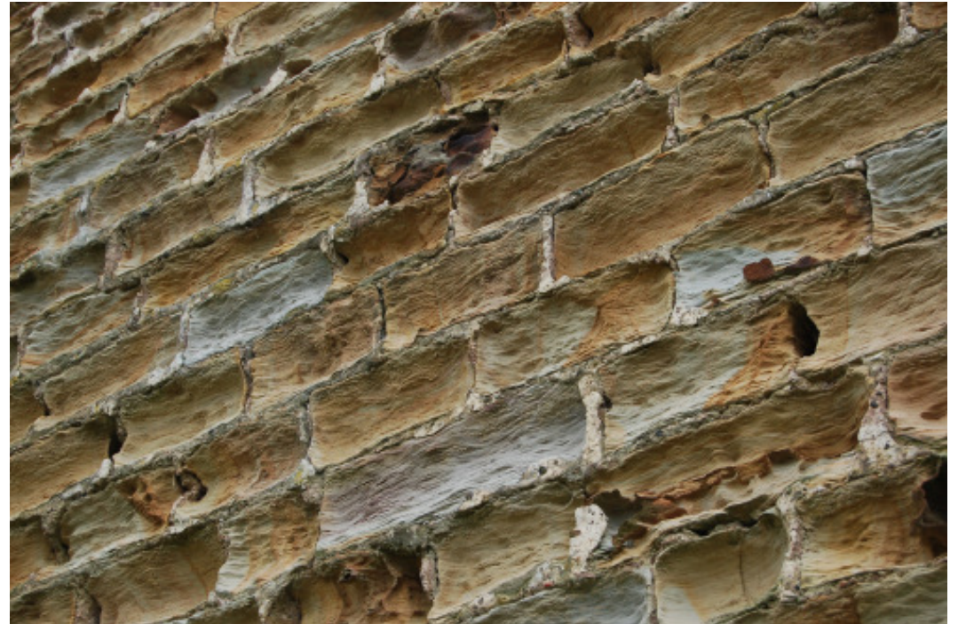
Weathering of the facing stone
