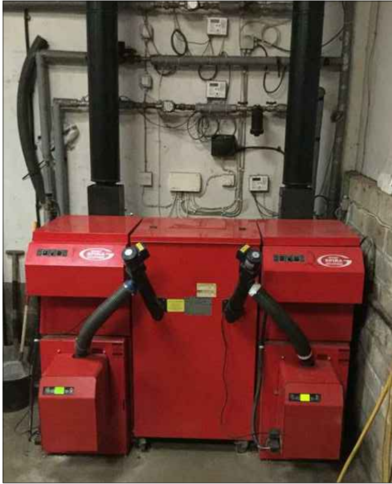
2x36kw Biomass Boilers
