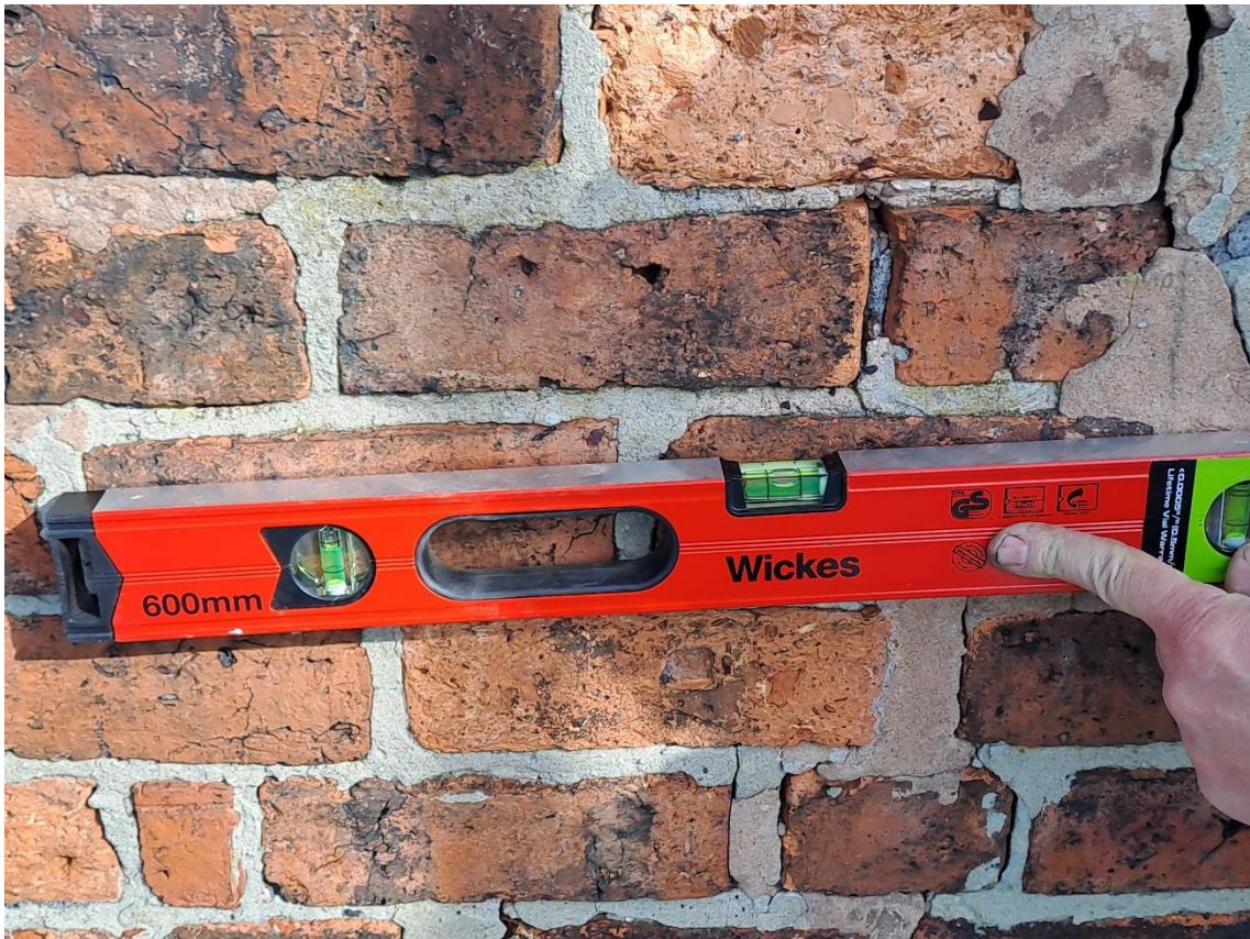
Front Elevation showing the significant out of level.
