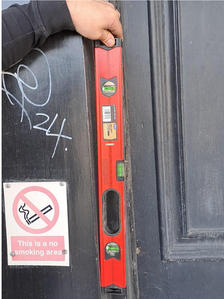
Front door reveal showing the significant out of plumb.
