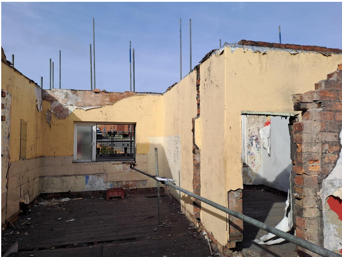
Internal view showing the significant out of level floor and cracking.
