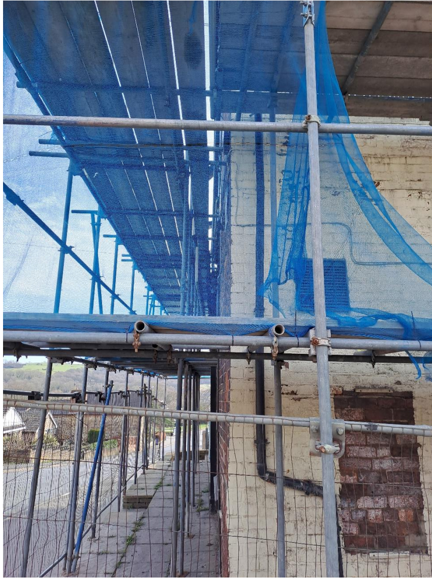
Front Elevation showing the significant out of plumb and bowing.
