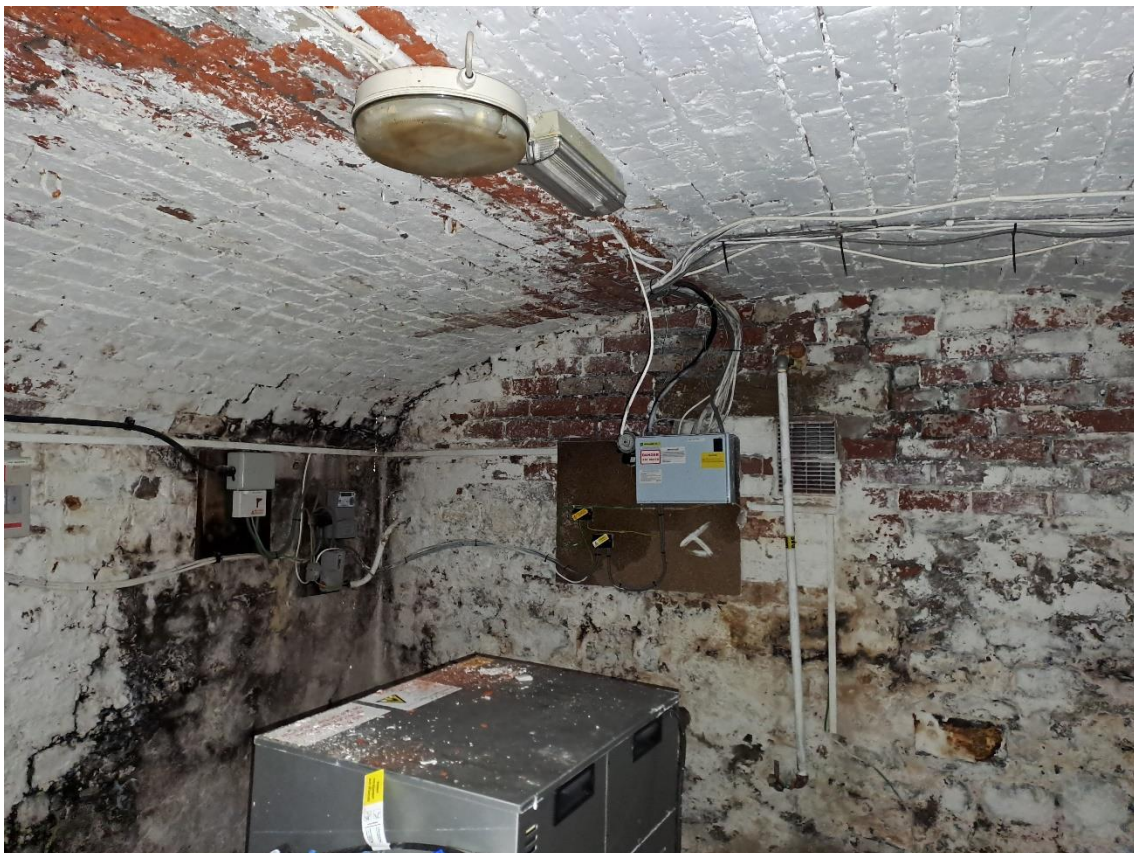
Basement view showing the flattened arch and damp
