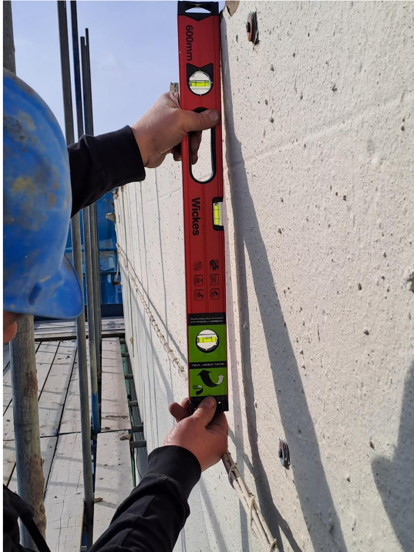
Side Elevation showing the significant out of plumb.
