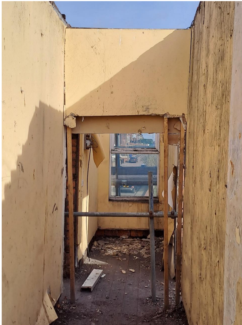
Internal corridor showing the significant out of plumb adjacent to the door and cracking.
