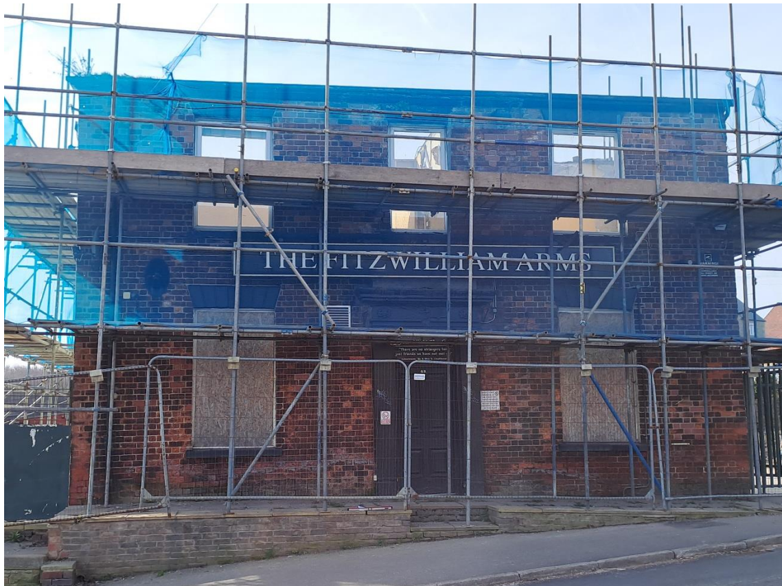
Front Elevation showing the extent of the tilt.
