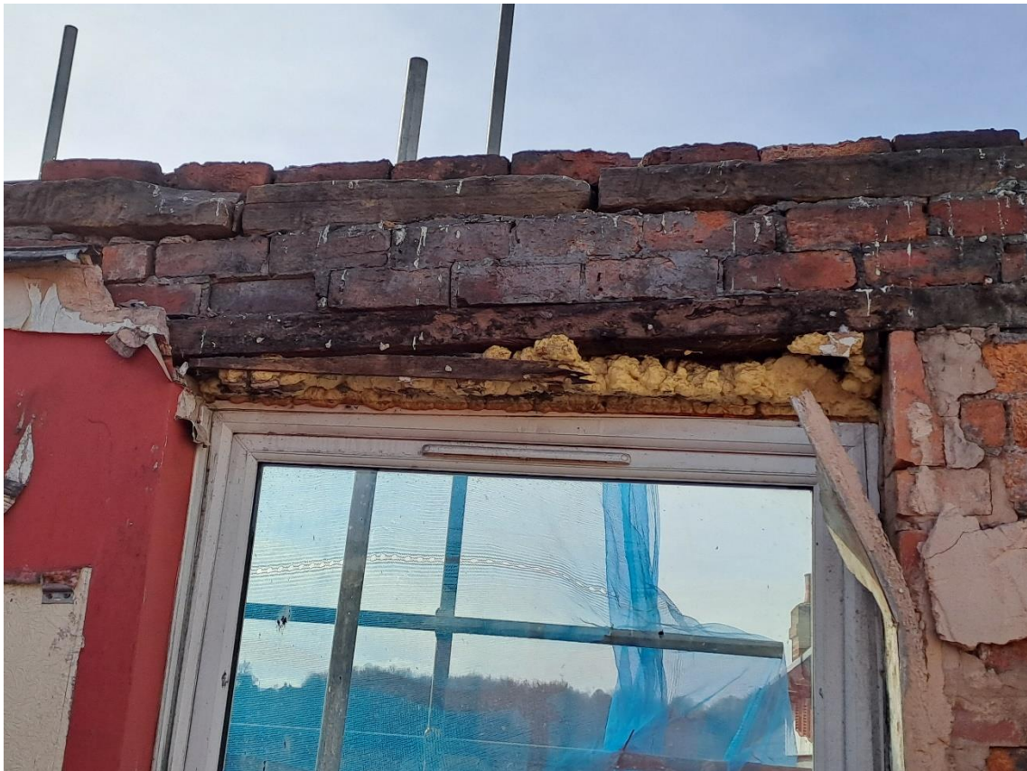
Internal Side Elevation window head showing the significant out of level.
