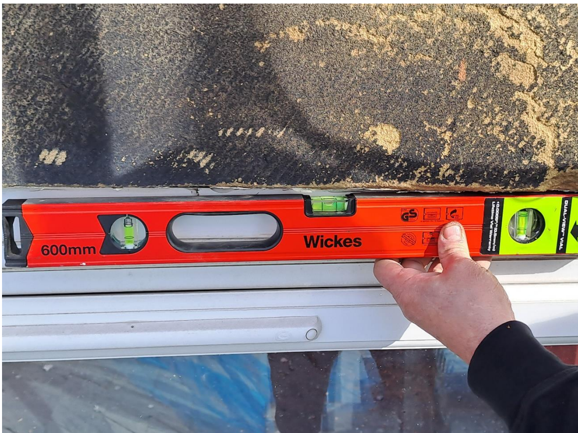
Front window head showing the significant out of level.
