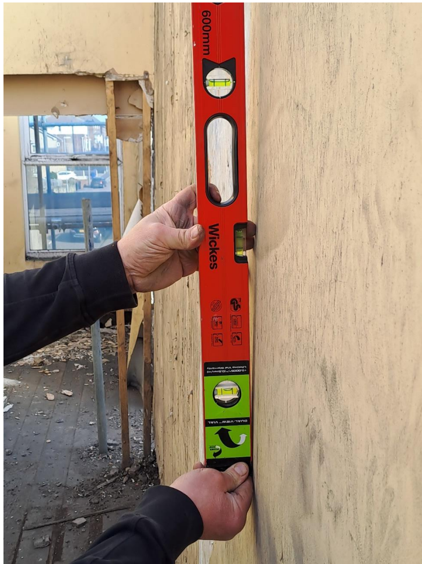
Internal wall showing the significant out of plumb.
