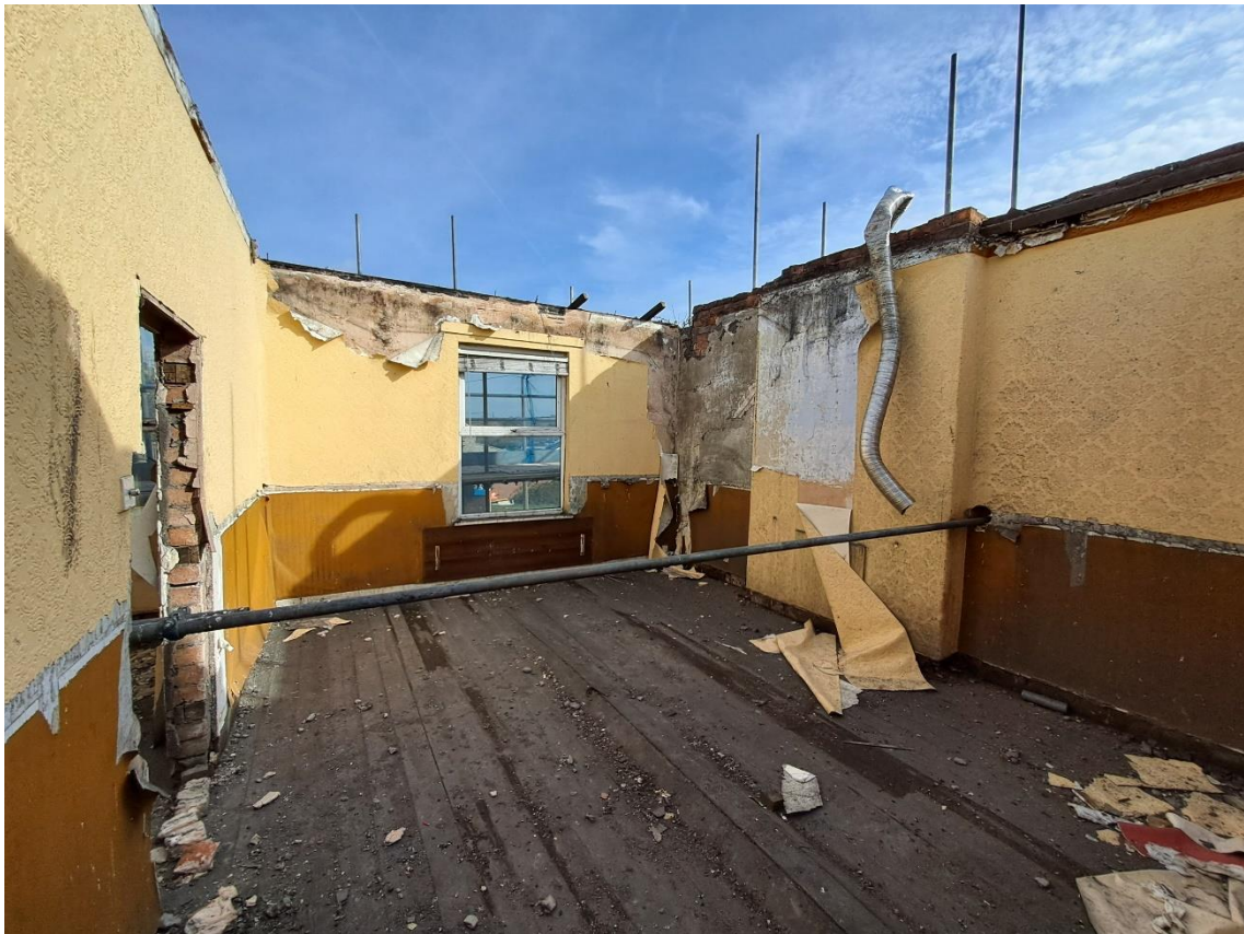
Internal view showing the significant out of level front window.
