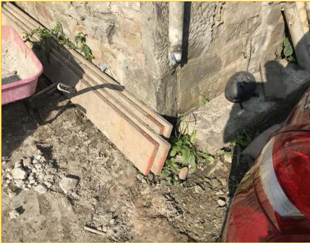
Photograph - 6 - Typical discharge to ground
