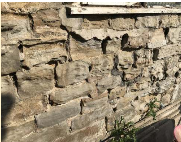
Photograph - 37 - Weathered masonry
