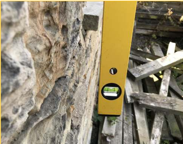
Photograph - 28 - Extent of tilt
