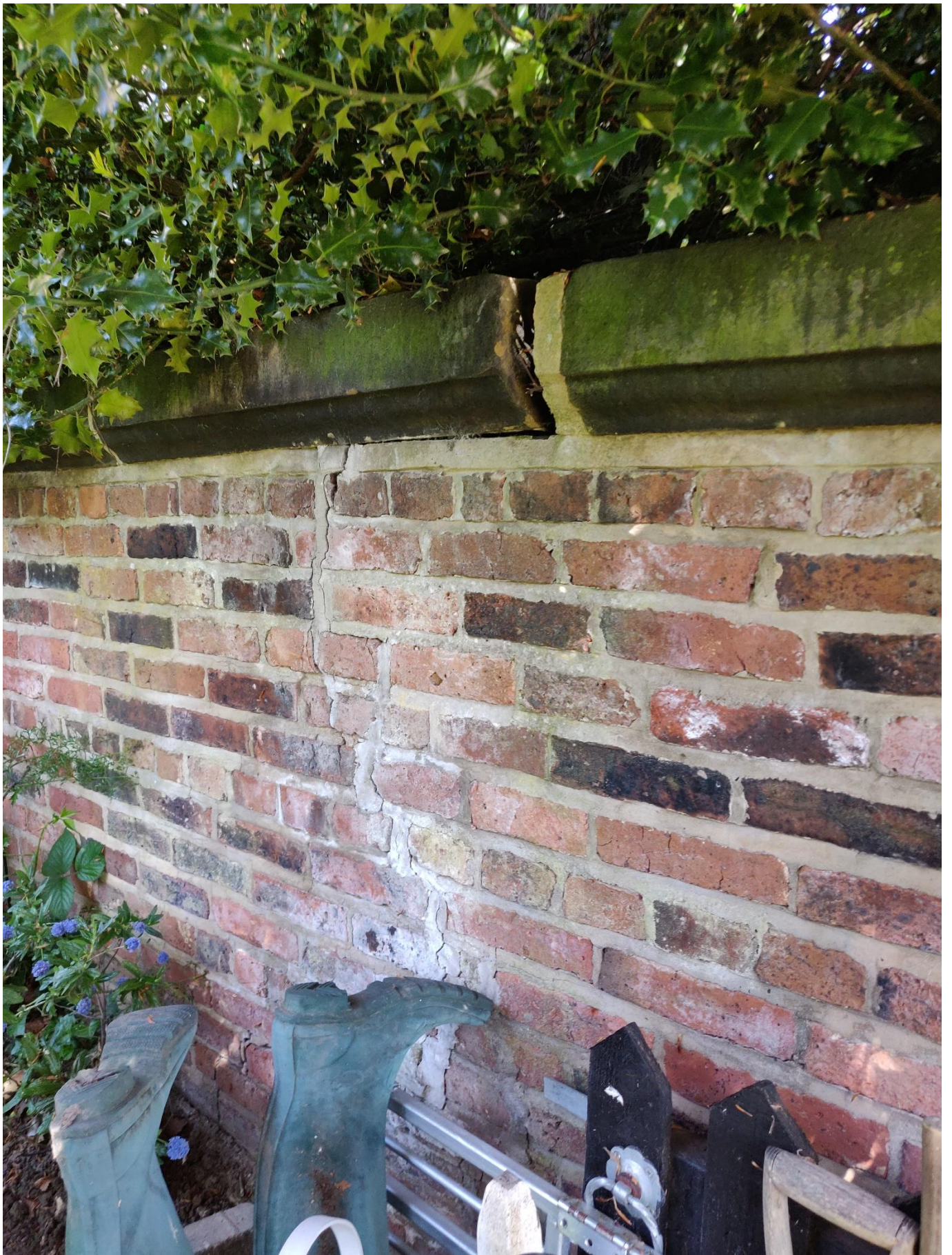
Photograph 2 – View of cracking close to movement in copings (note prevent point repair of crack and wider joints)
