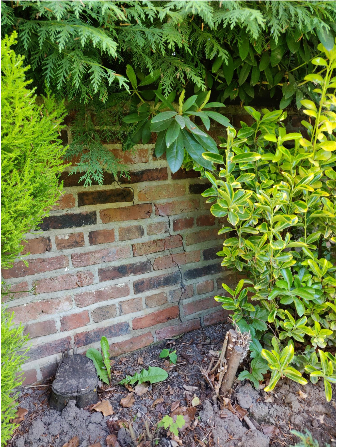
Photograph 3 – View of cracking 1.50m from Copper Beech Tree
