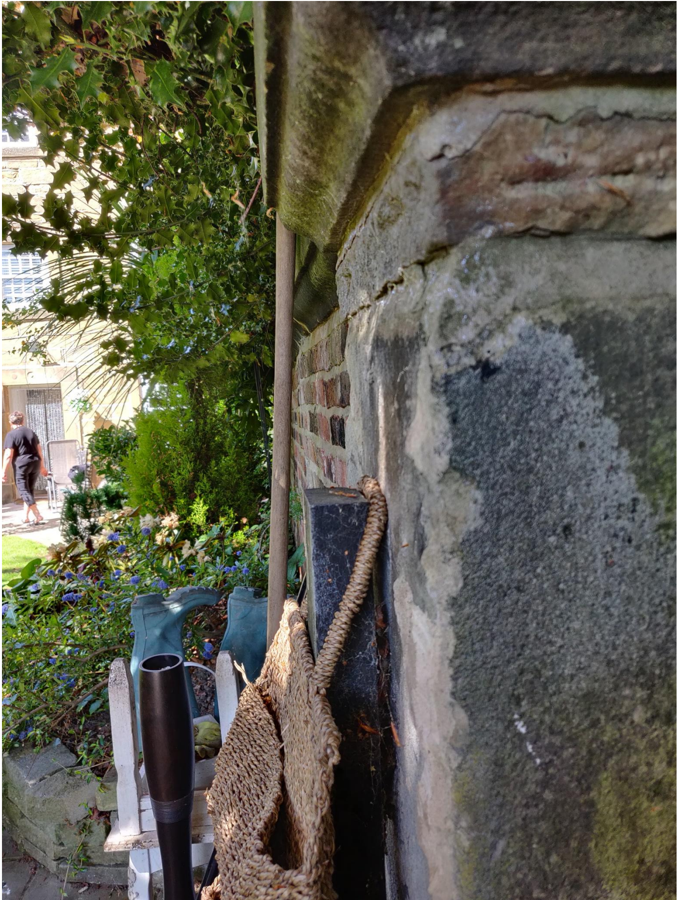
Photograph 4 – View along wall showing outward lean into neighbouring garden
