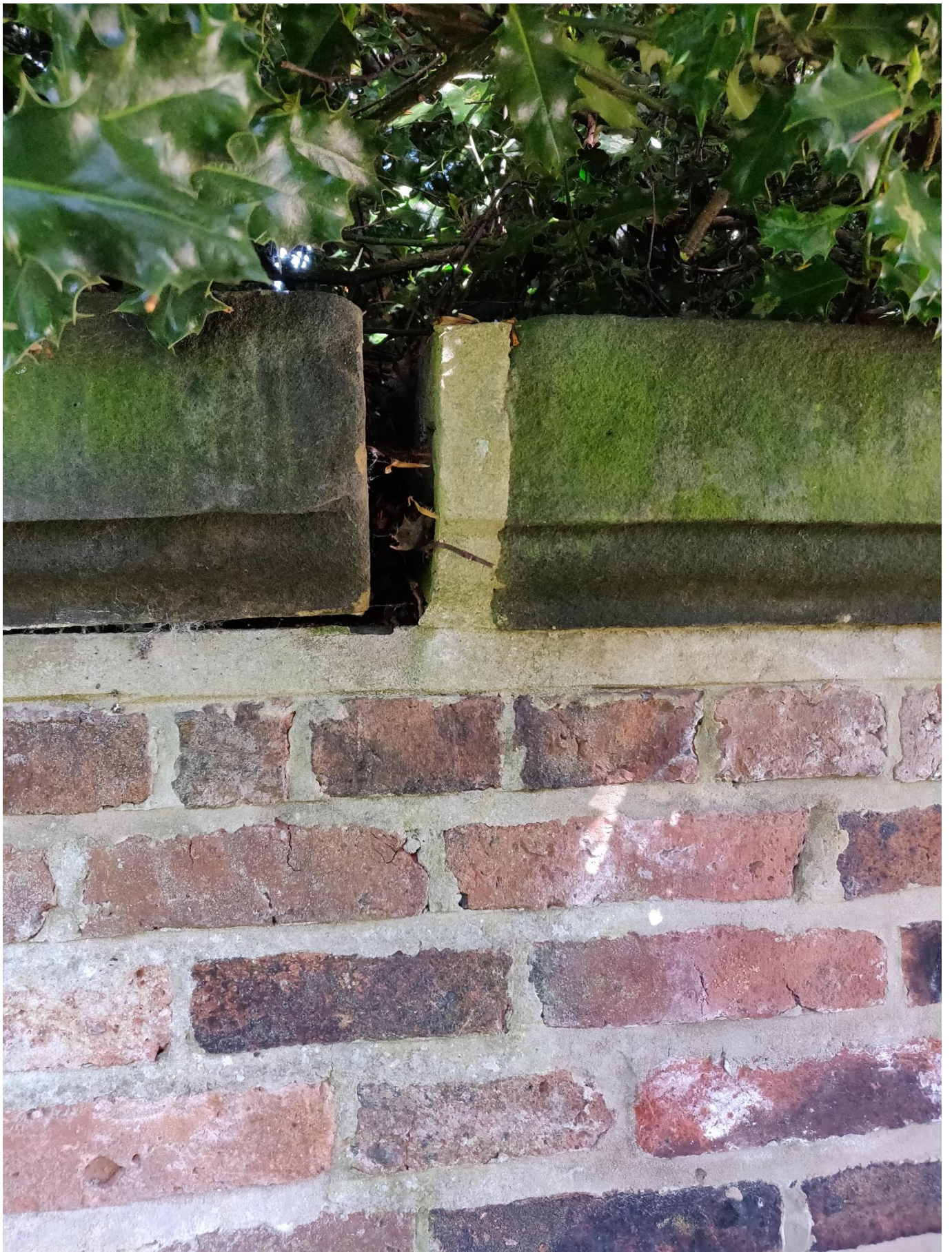
Photograph 1 – View of lateral and uplift movement of coping stone adjacent to Copper Beech Tree
