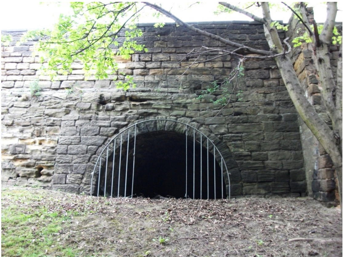
Plate 6: Blocked Culvert under Old Mill Lane
