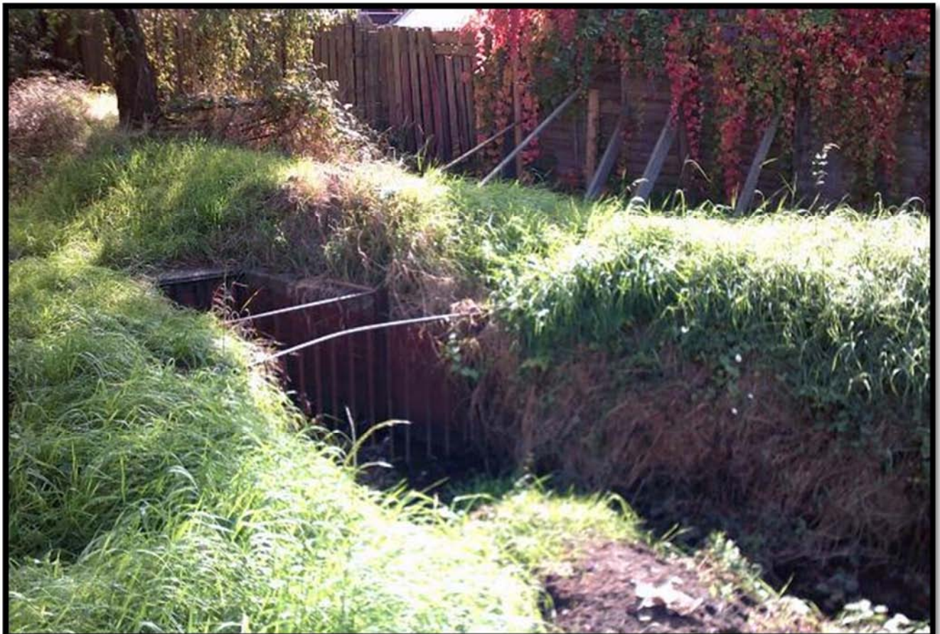
F: The site watercourse had been culverted in the southeast of the site.
