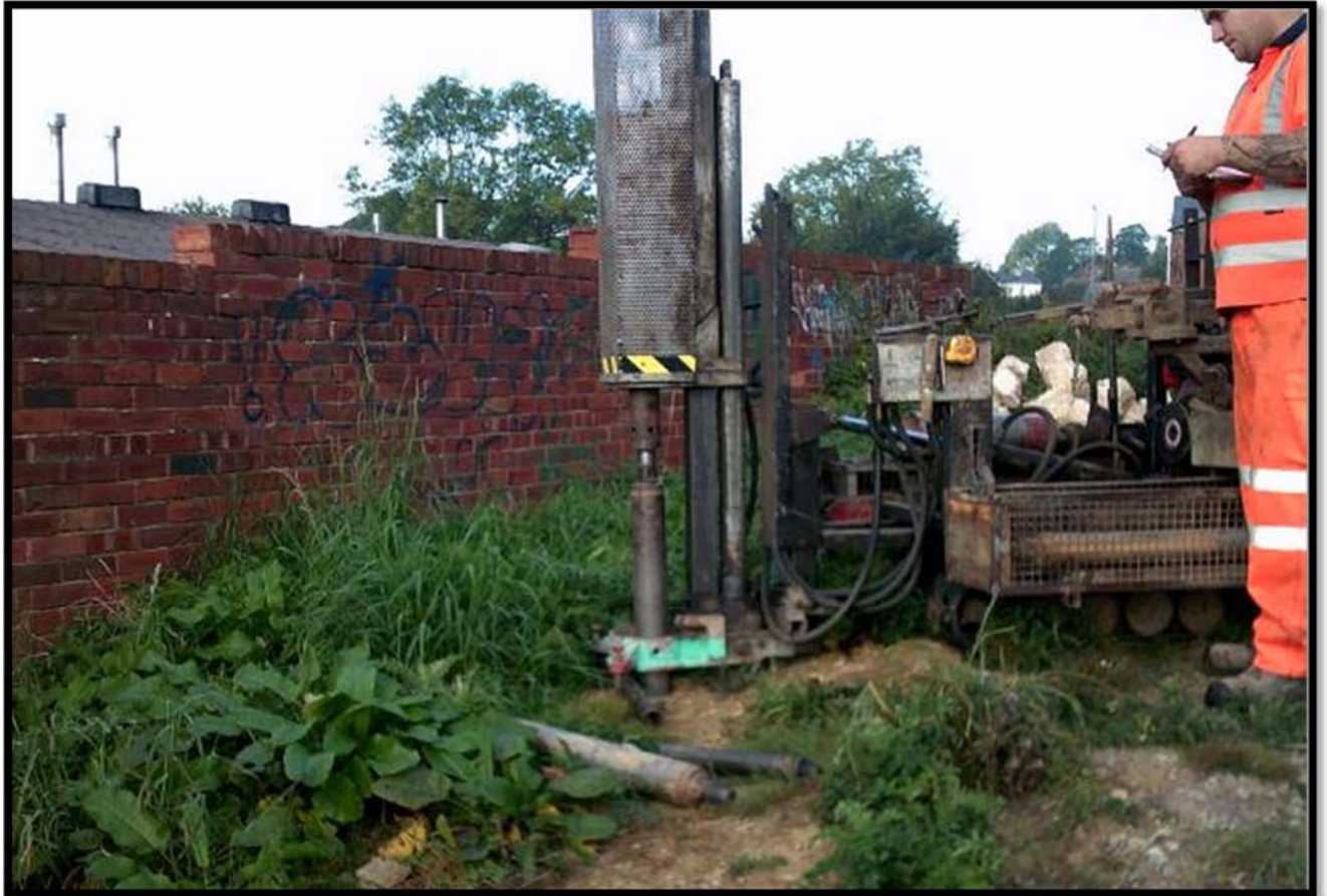
A: Window sample borehole WS01 was located behind a retaining wall at the northeast corner of the site.
