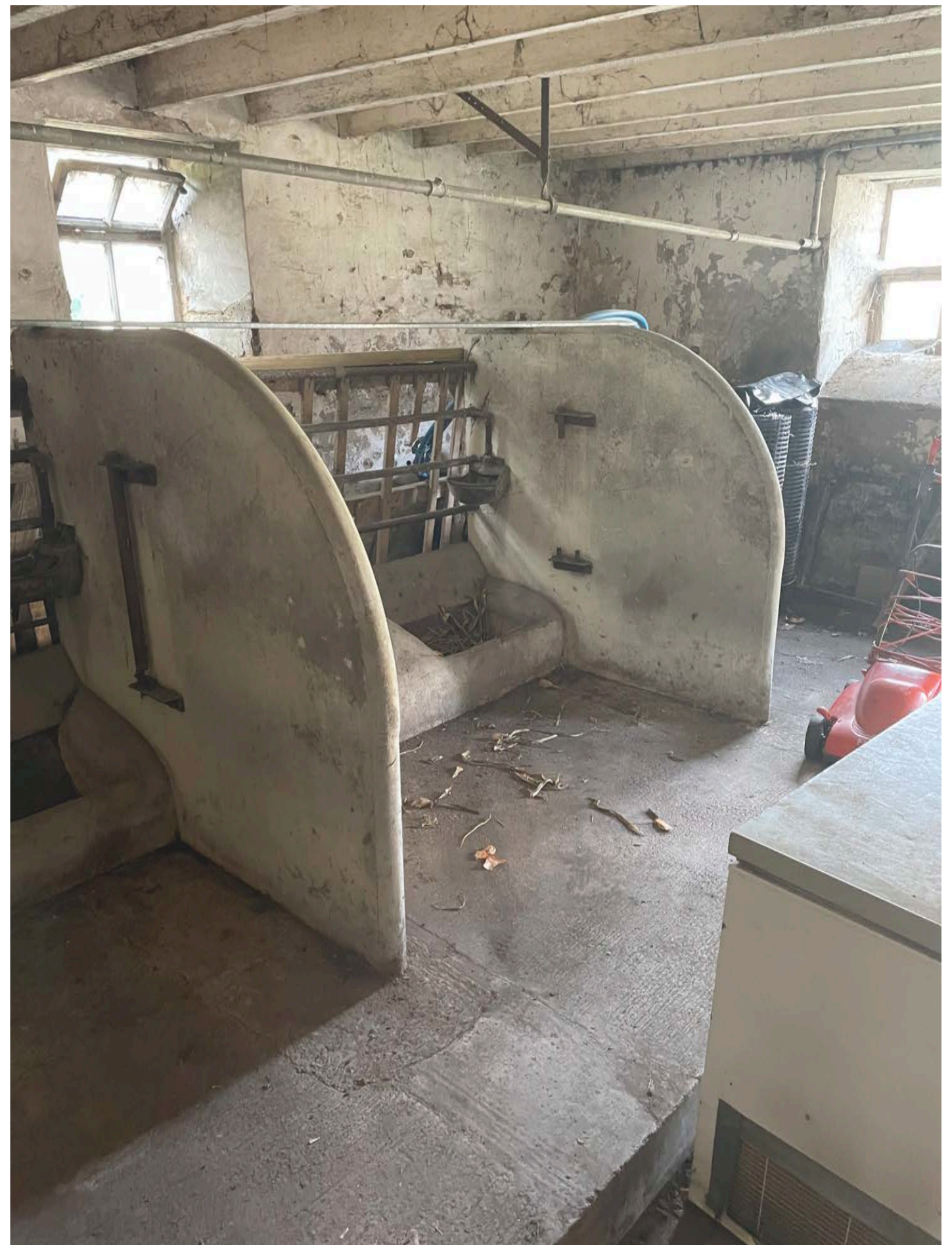
Photo Ref: E09 View of Nether Mill Barn (Internal Detailing Cattle Feeding Station)
