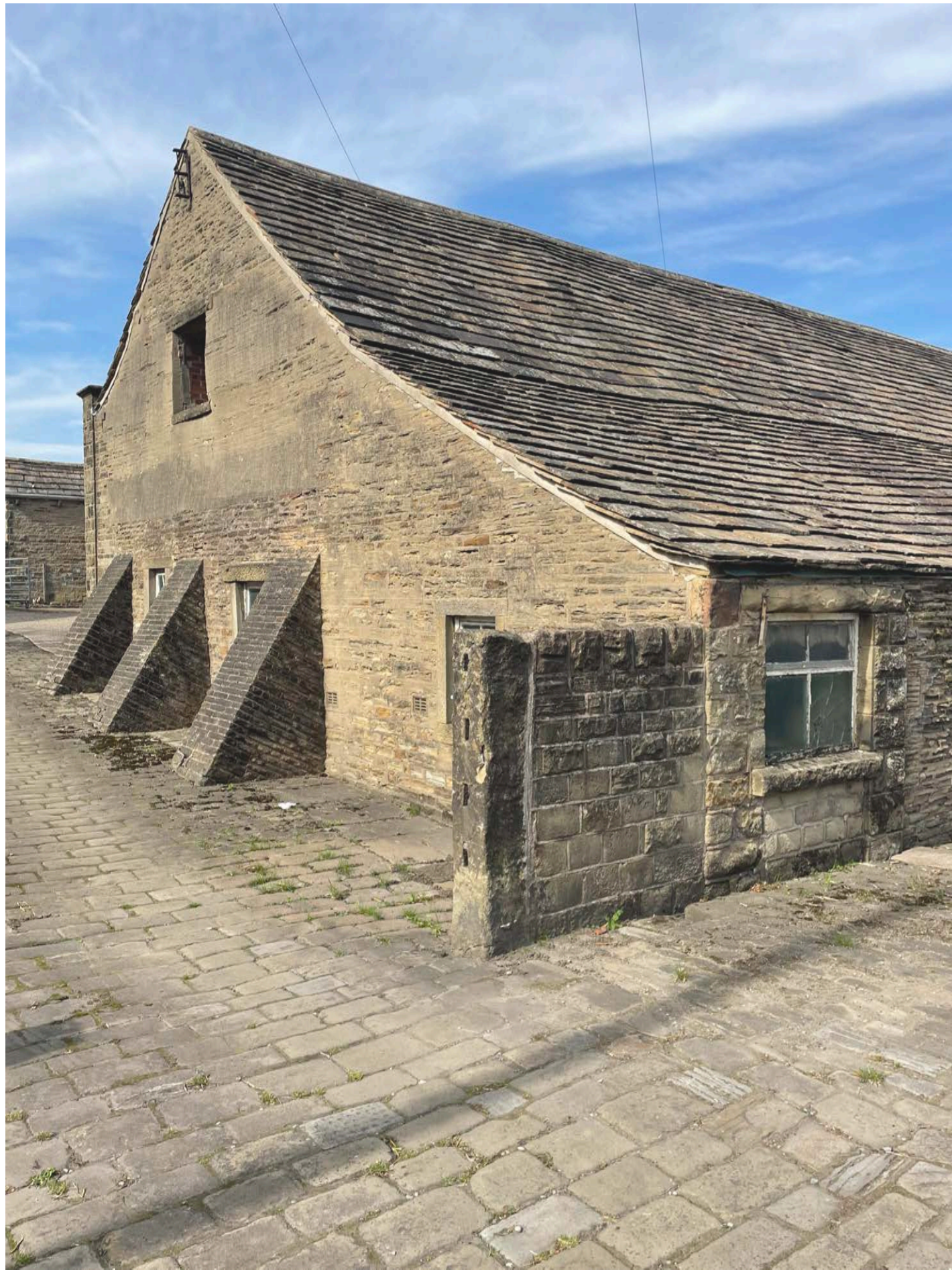
Photo Ref: E04 View of Nether Mill Barn (Side Elevation) from Vehicular Access
