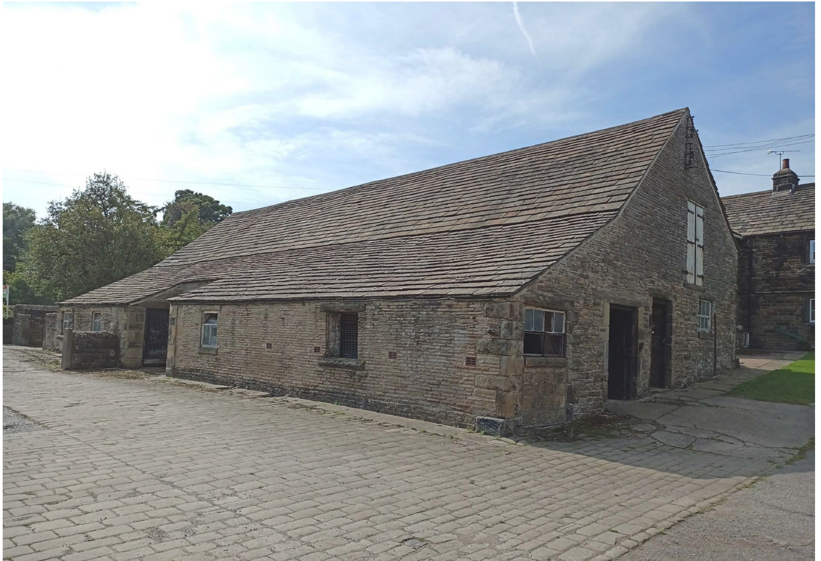
Photo Ref: E03 View of Nether Mill Barn (Primary Elevation) from External Area
