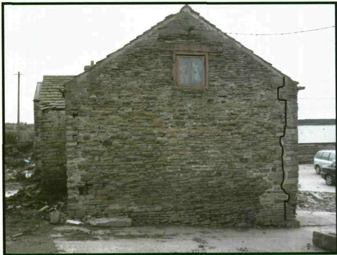
Photograph 4 – North Elevation (Gable) Crack highlighted
