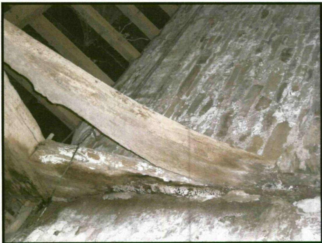
Photograph 13 – Wet rot to timber leg
