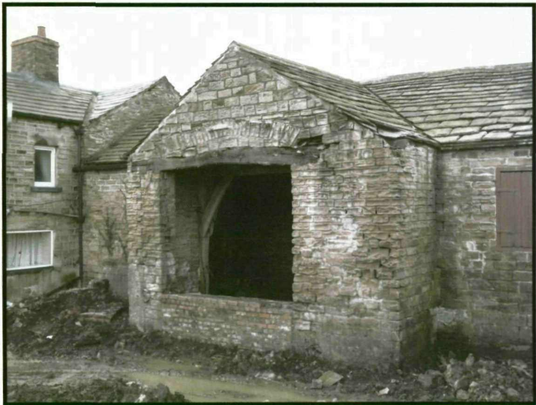
Photograph 8 – East Elevation showing damage to gable at eaves
