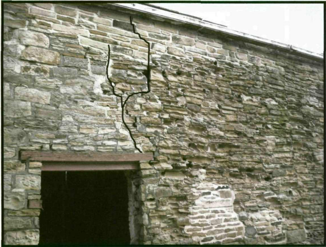
Photograph 3 – West Elevation cracking shown highlighted above doorway
