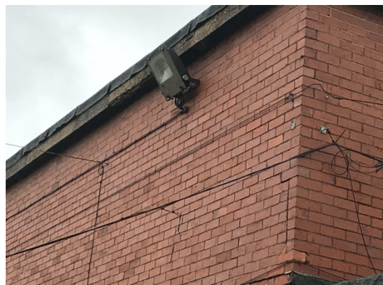
Image 20: Lifted felt on western side of Building 1
