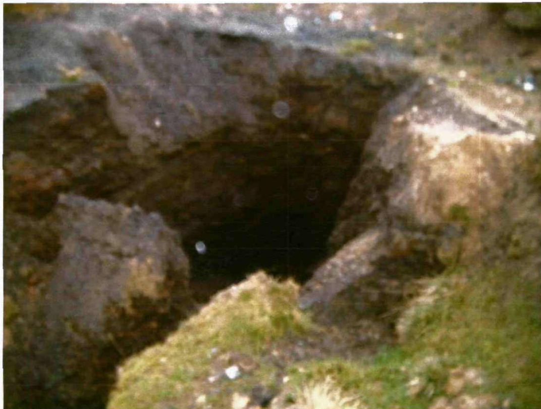
Photograph number 6 showing the old adit and mine tunnel for the Halifax Hard Bed. The tunnel is open and the ground is collapsing around the entrance. Surface Water Point SW3.
