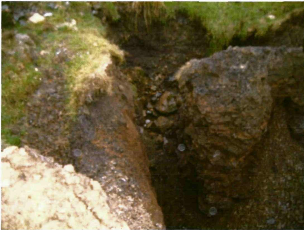
Photograph Number 9 showing the collapsed ground around the old roadway and adit being eroded by the surface water run off over the site.
